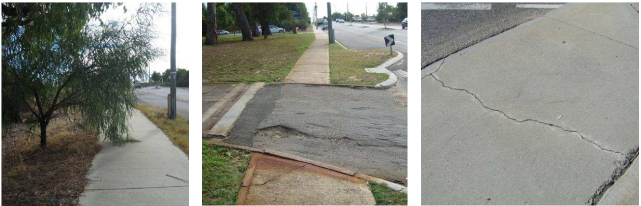
Figure 6 : Poor maintenance and design of footpath
