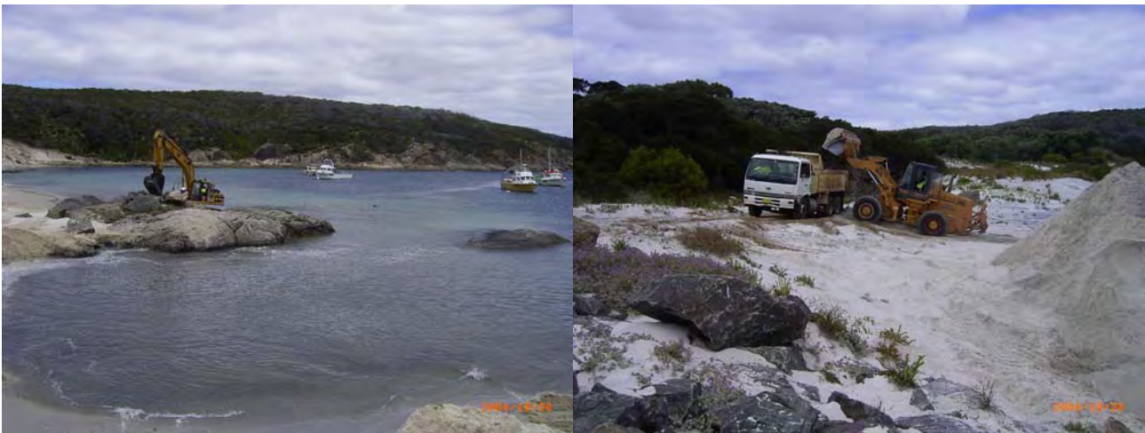
Figure 13: Two photographs from the 26 th October 2004 showing the excavation of sand from the boat ramps at the eastern end of the beach. Maintenance similar to this has been conducted at least once a year for several years to ensure the boat ramp can be used at peak holiday periods over summer.
