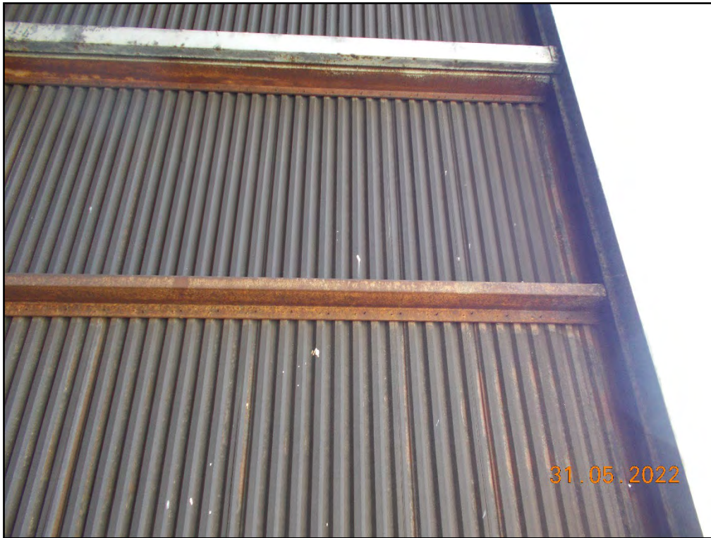
Photograph 63 Surface Corrosion of Girts
