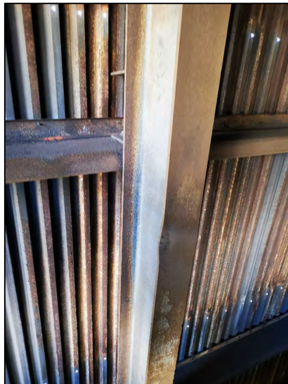
Photograph 36 Impact Damage of Column
