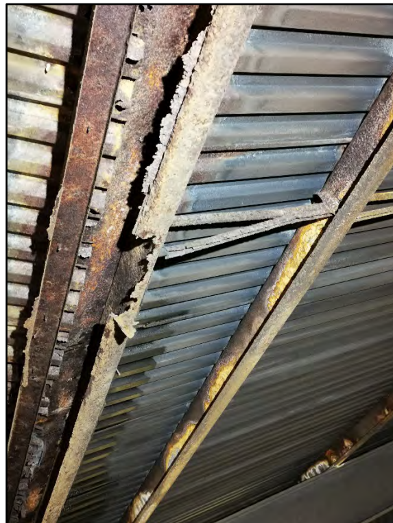
Photograph 139 Deterioration of Purlin
