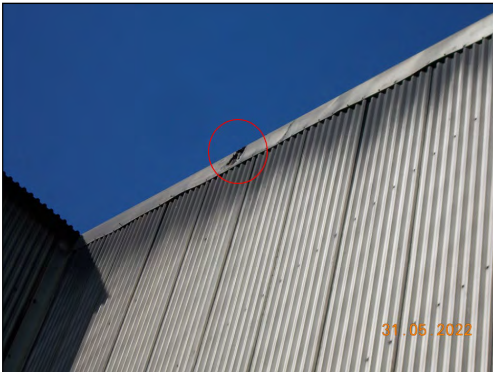
Photograph 53 Deterioration Observed to the Flashing North Side of Shed 7
