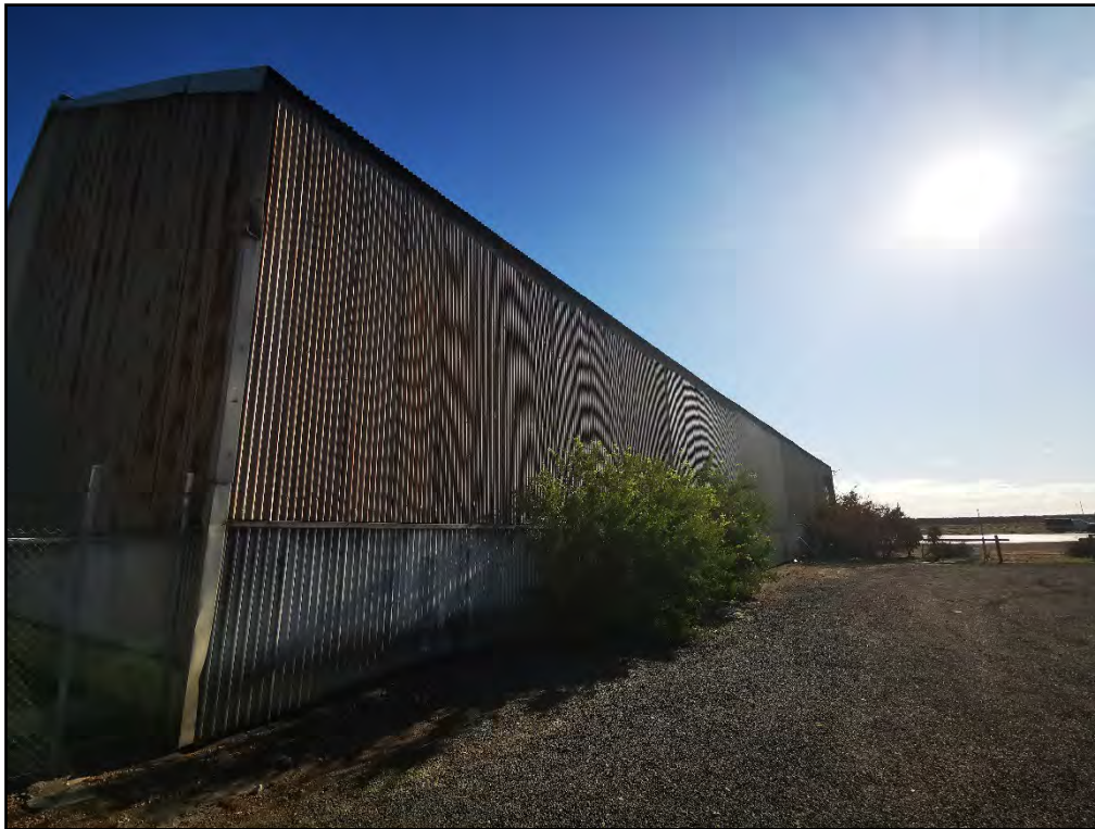
Photograph 8 Wall Sheeting East Side Minimum Damage
