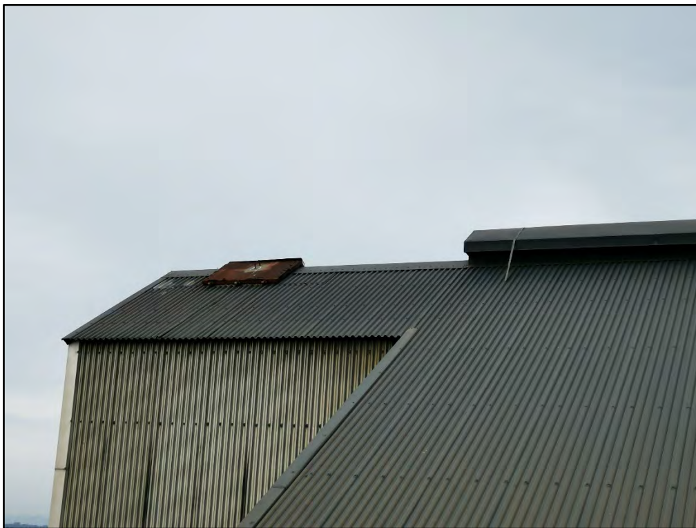
Photograph 55 Corrosion of Access Door
