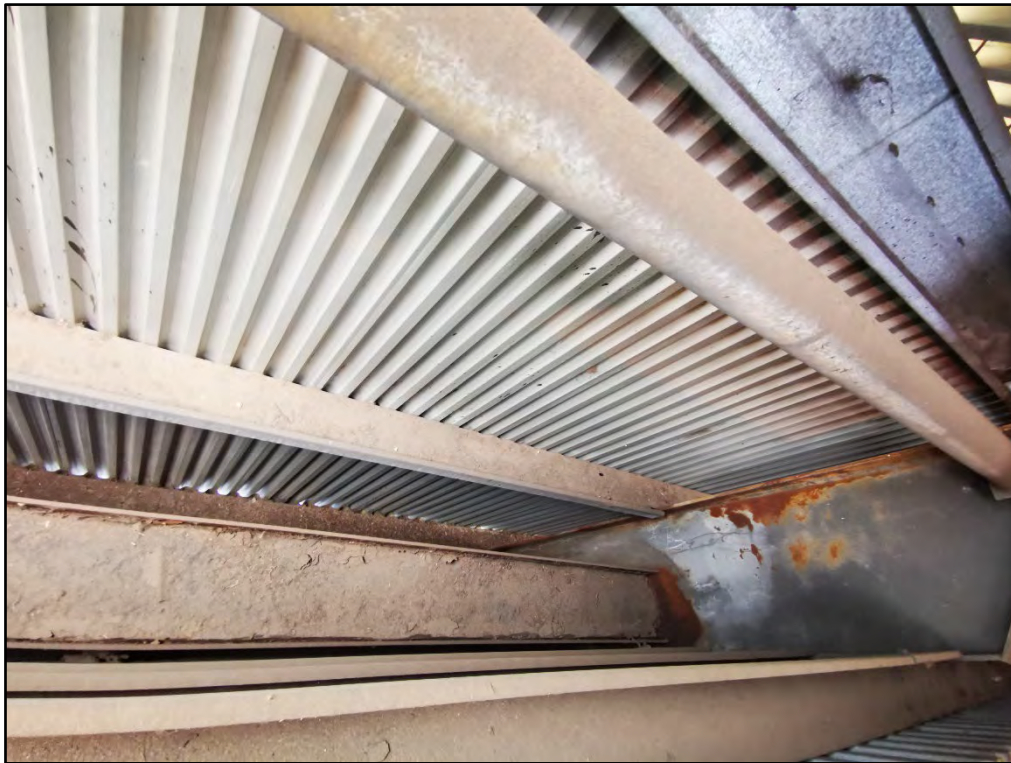
Photograph 156 Surface Corrosion of Column
