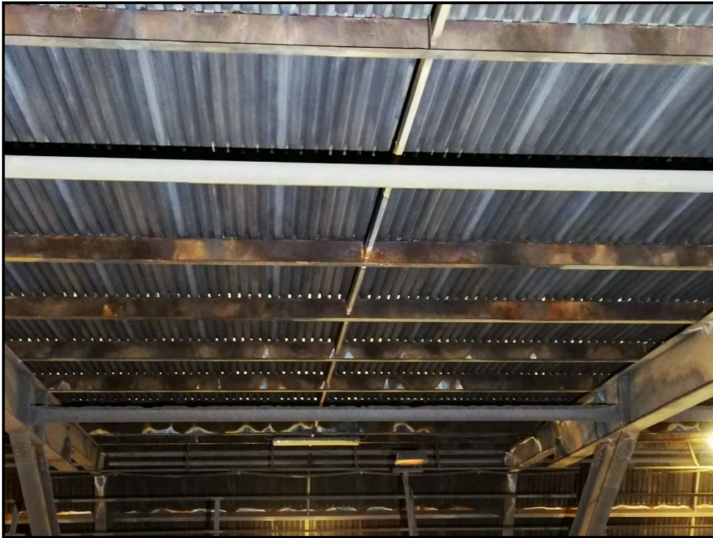
Photograph 92 Surface Corrosion of Purlins and Rafters
