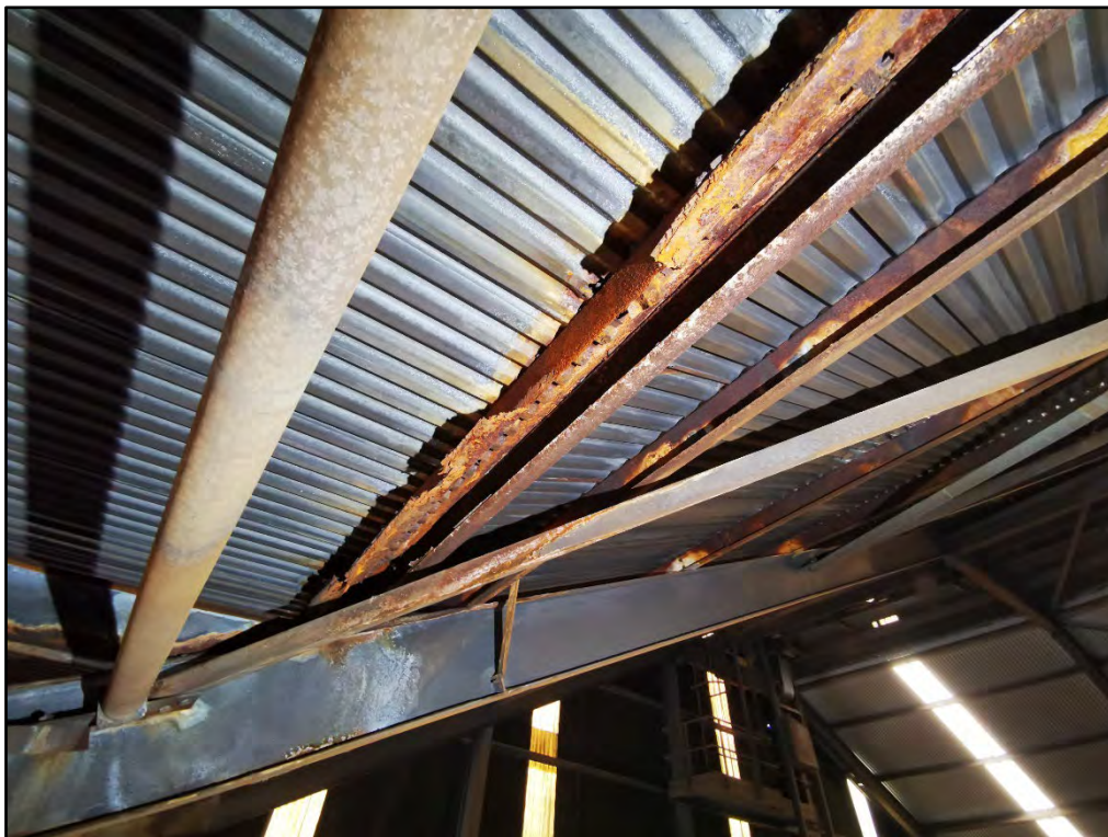
Photograph 141 Daeteriorated Purlin due to Corrosion
