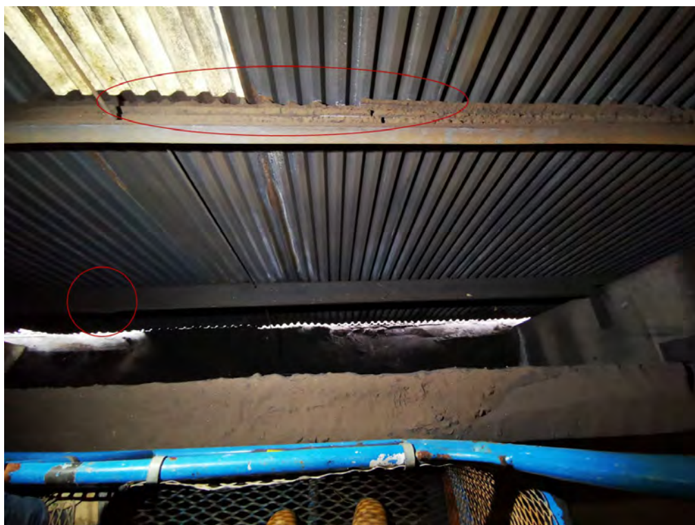
Photograph 103 Sectional Loss and Damage of Girt Due to Product Deposit
