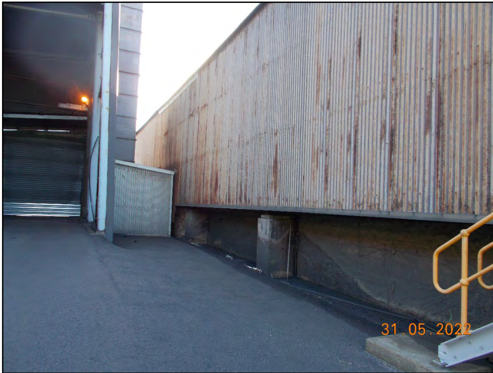
Photograph 6 Corrosion on Wall Sheeting
