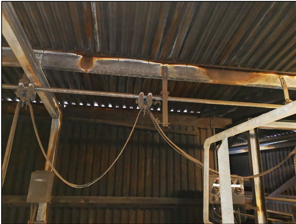
Photograph 168 Sectional Loss of Fascia Purlin and Surface Corrosion of Purlins and Girts
