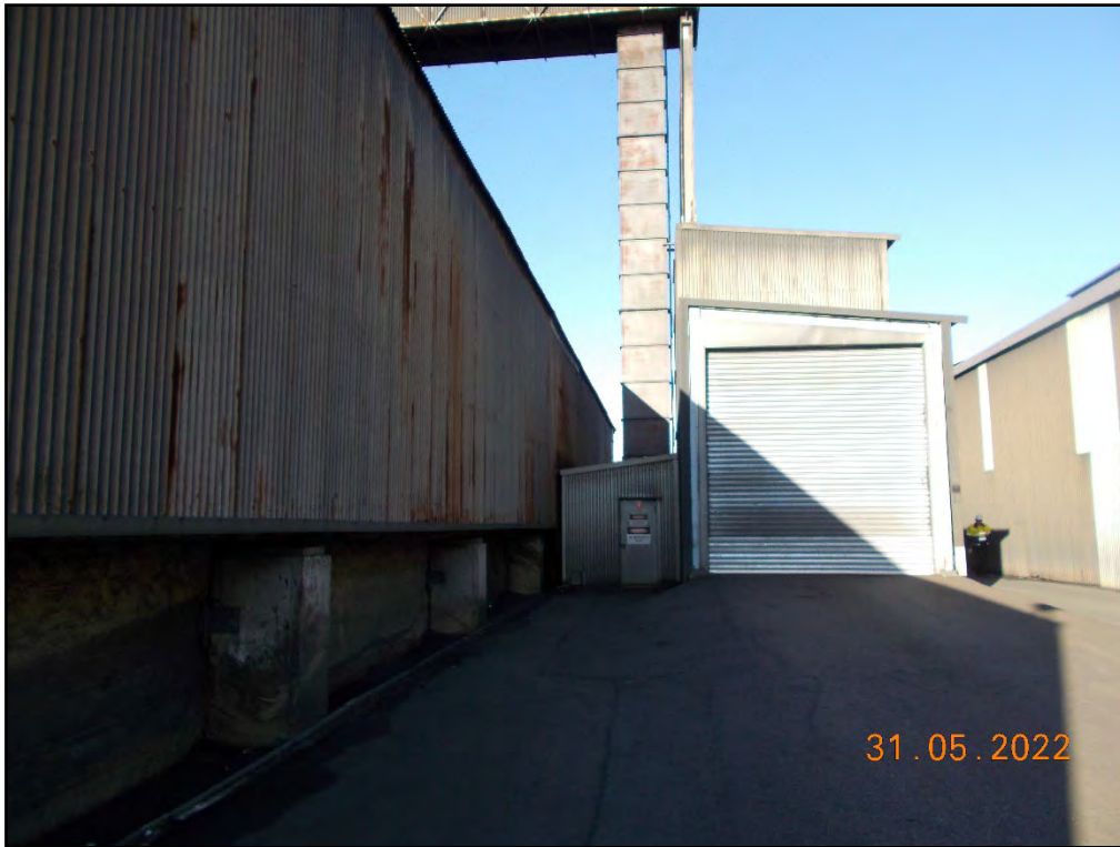
Photograph 4 Corrosion on Wall Sheeting
