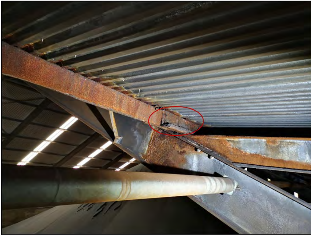
Photograph 136 Delamination of Purlin due to Corrosion
