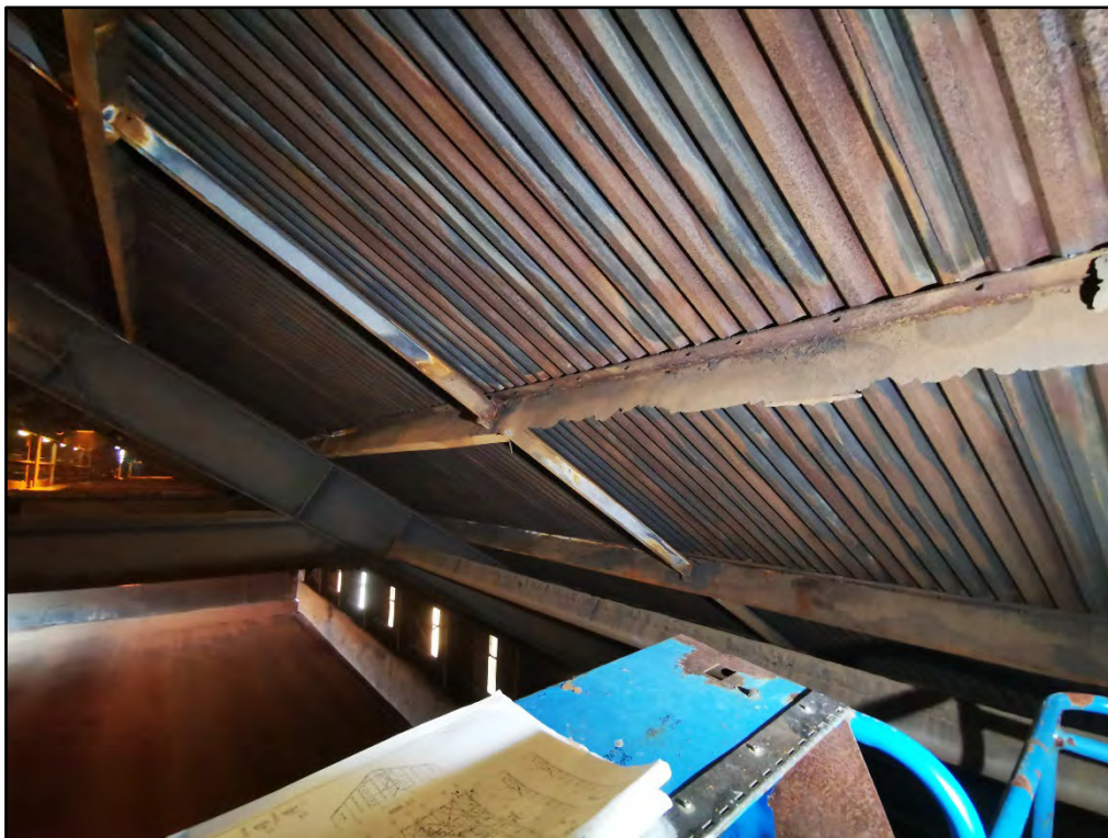
Photograph 99 Sectional Loss of Purlin
