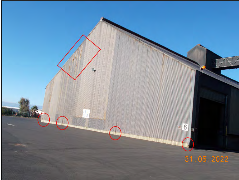
Photograph 2 Impact Damage Observed During Inspection and Corrosion of Sheeting
