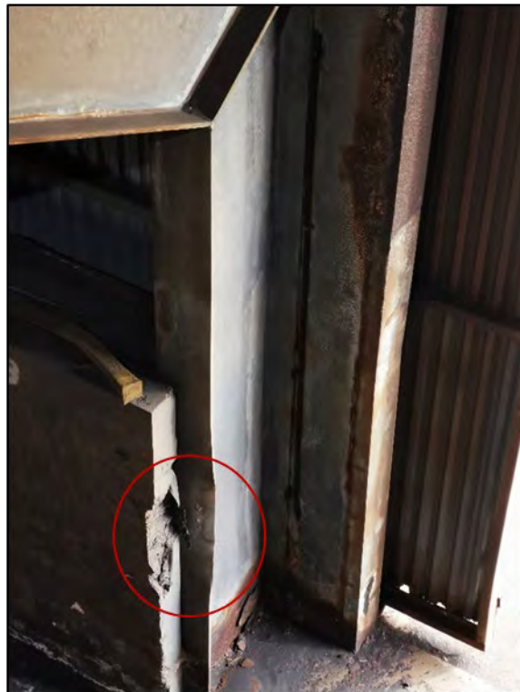
Photograph 137 Damaged Concrete Wall and Impact damage to Column Bay H-3
