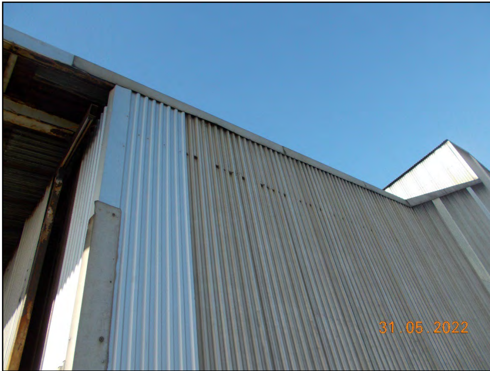
Photograph 126 Corrosion of Door Frame
