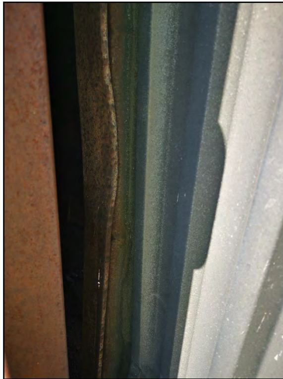
Photograph 128 Damage Due to Impact
