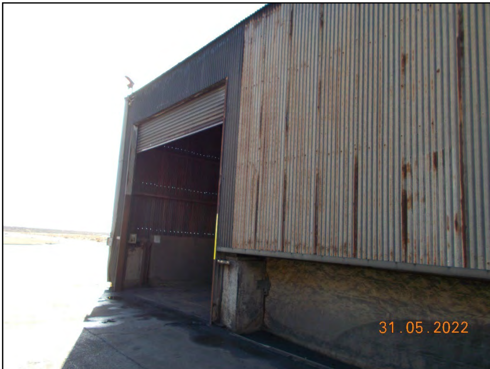
Photograph 3 Corrosion on Wall Sheeting
