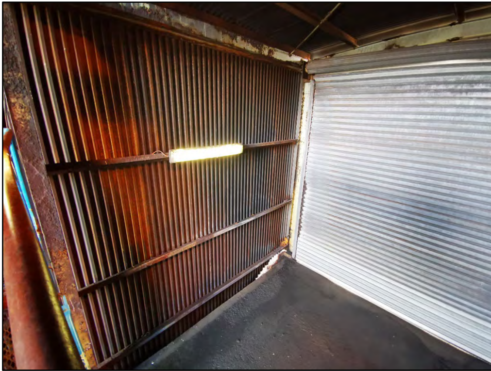
Photograph 18 Corrosion of Wall Girts and Sheeting
