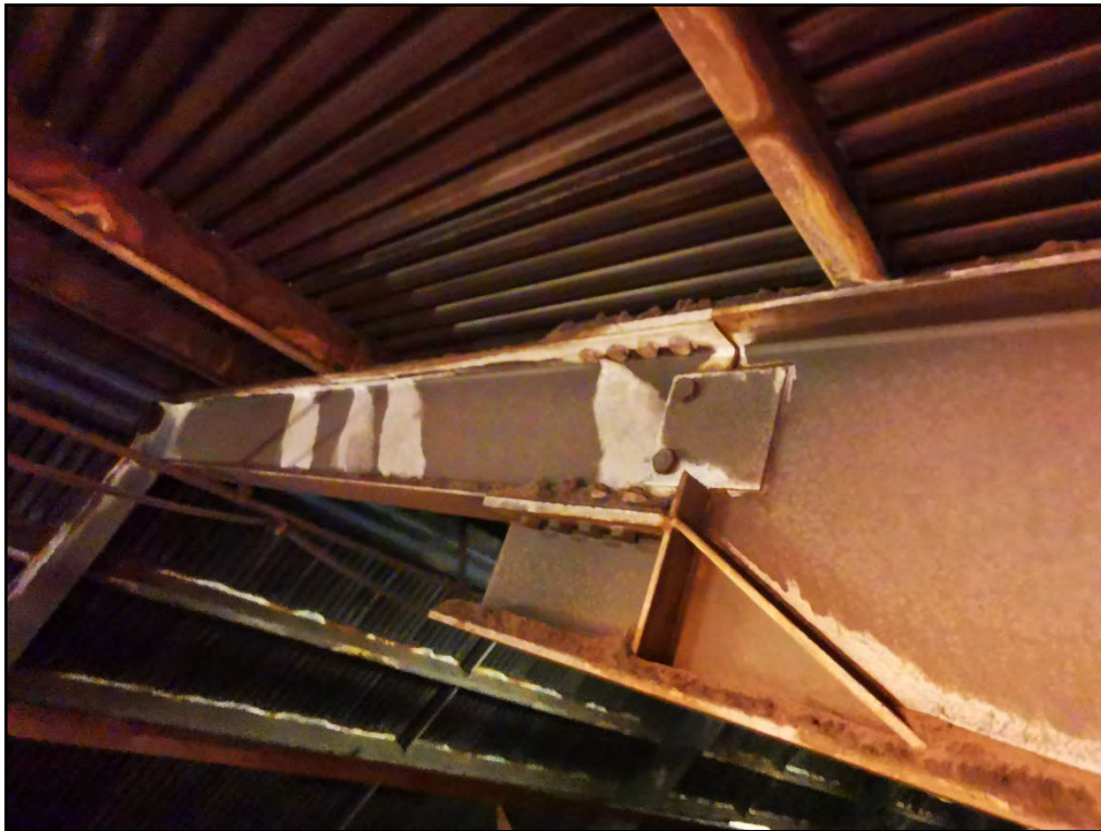
Photograph 84 Surface Corrosion of Rafter Due to Water Leakage and Product Deposit
