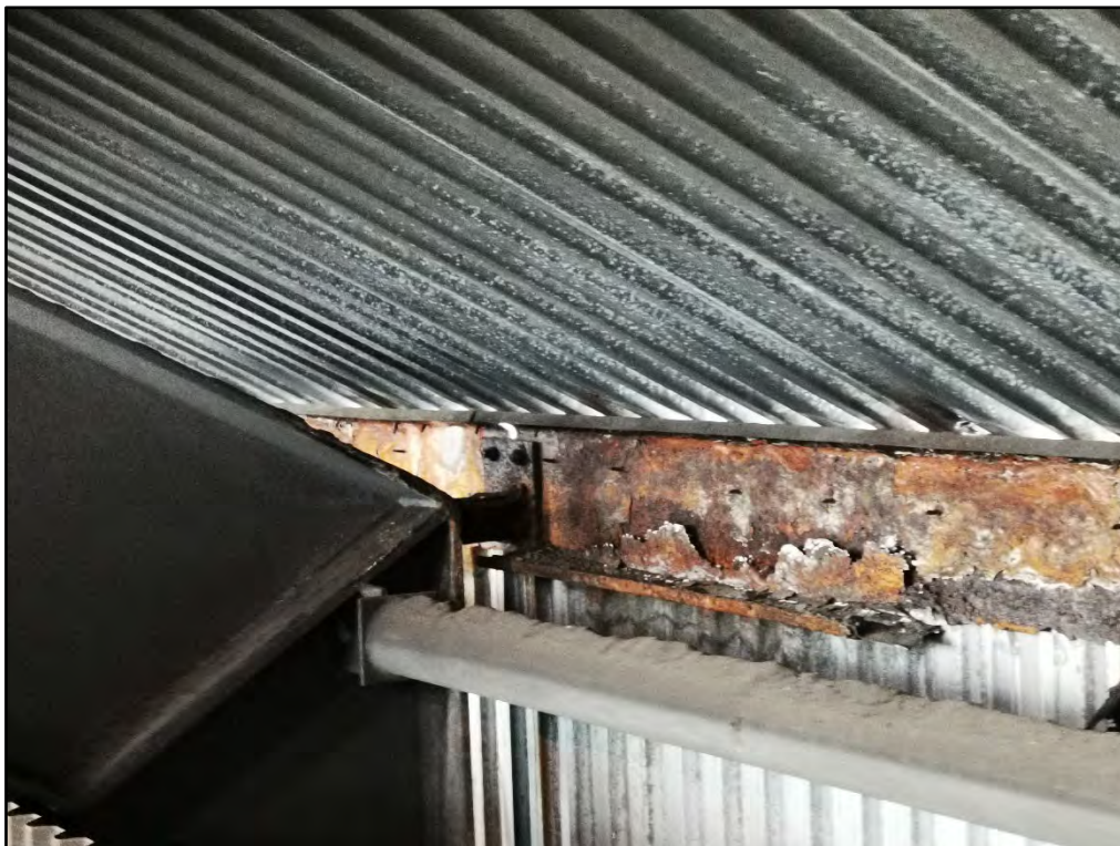
Photograph 153 Deterioration to Fascia Purlin due to Corrosion
