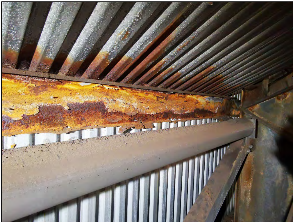
Photograph 143 Corroded Fascia Purlin
