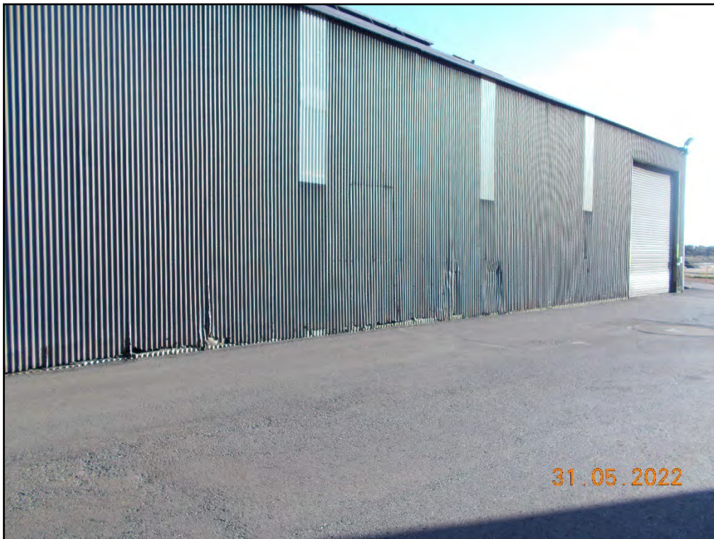
Photograph 45 Impact Damage and corrosion Observed
