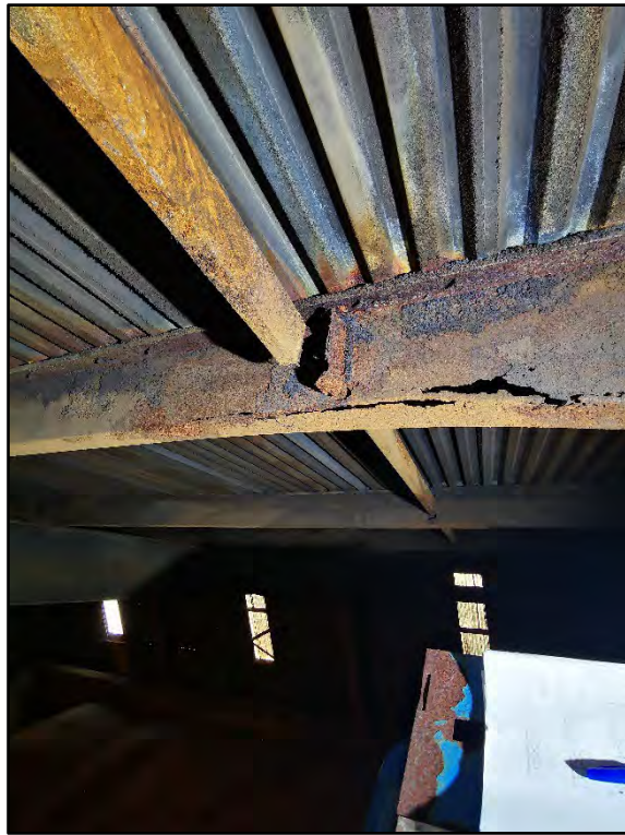
Photograph 98 Failure of purlin and bridging Due to Corrosion
