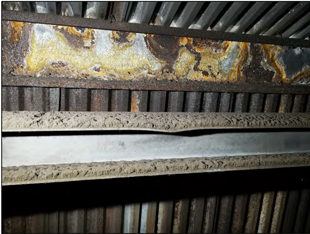
Photograph 33 Top Flange of Beam Damaged due to Impact
