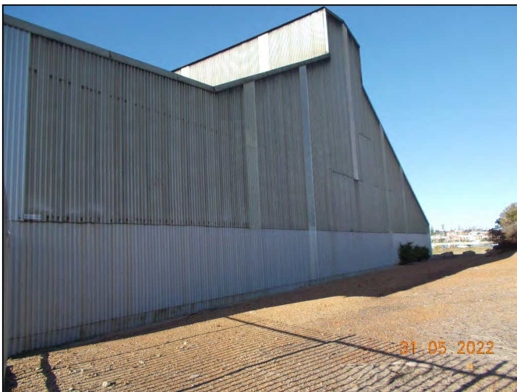
Photograph 127 Corrosion of Bolts
