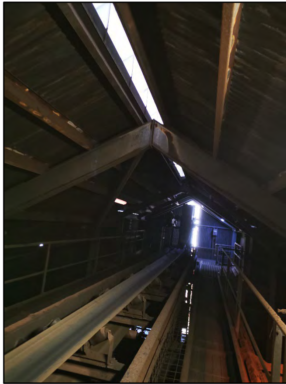
Photograph 120 Surface Corrosion of Purlins on Conveyor and Walkway
