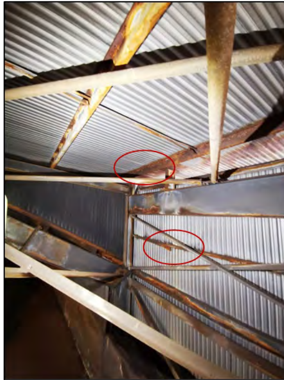
Photograph 138 Deteriorated Girts, purlins due to Corrosion and Surface Corrosion of Beams and Columns
