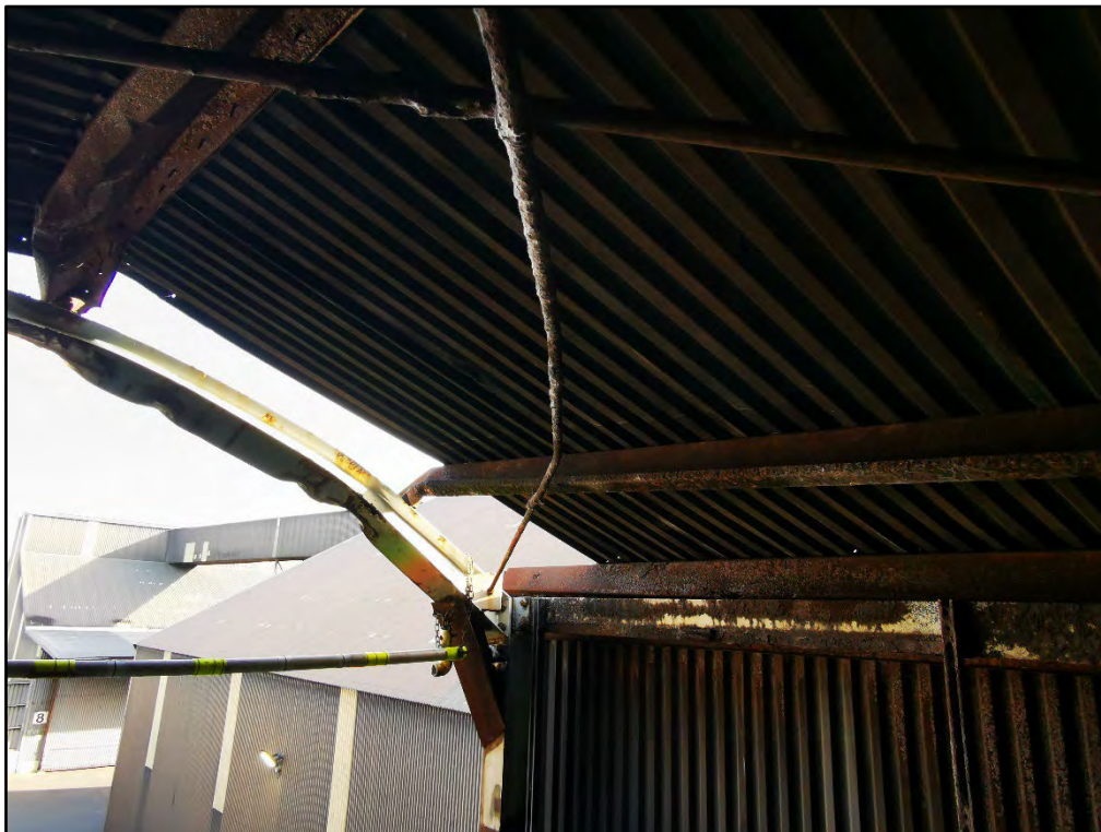
Photograph 13 Damage to Purlins, Bracings and Roof Sheeting Due to Impact
