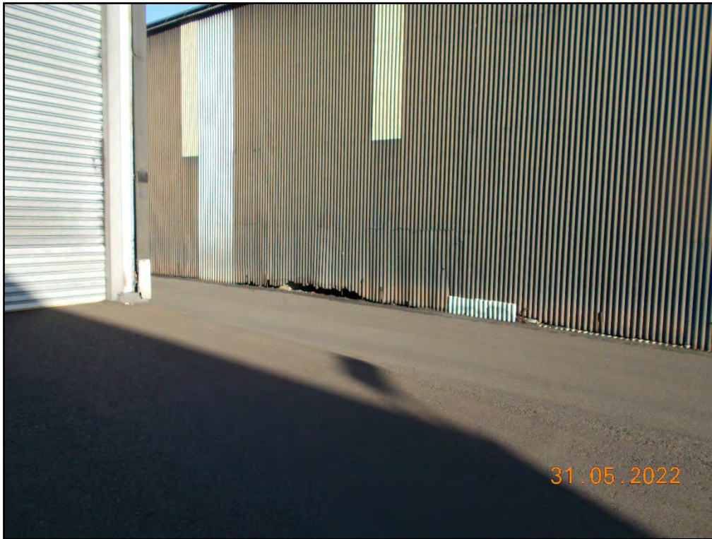
Photograph 46 Corrosion Deterioration at the Bottom of the Sheet
