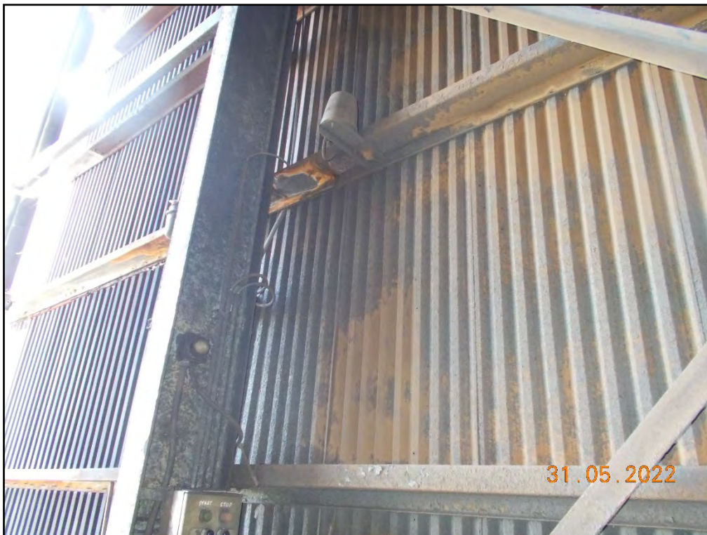
Photograph 66 Heavy Corrosion of Girts
