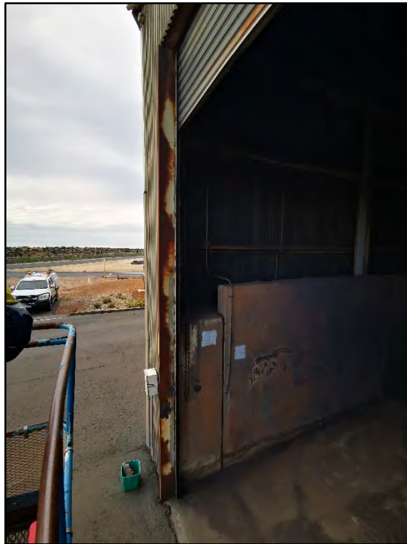
Photograph 114 Surface Corrosion of Door Frame
