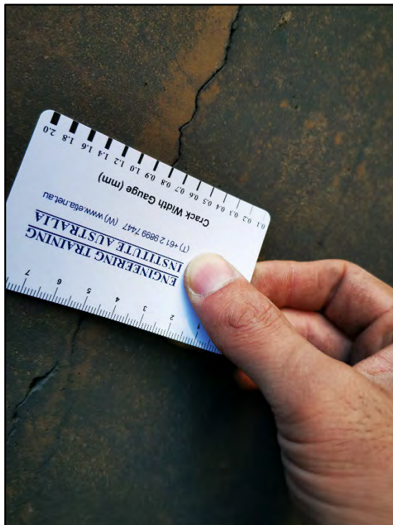
Photograph 115 Surface Crack on the Wall
