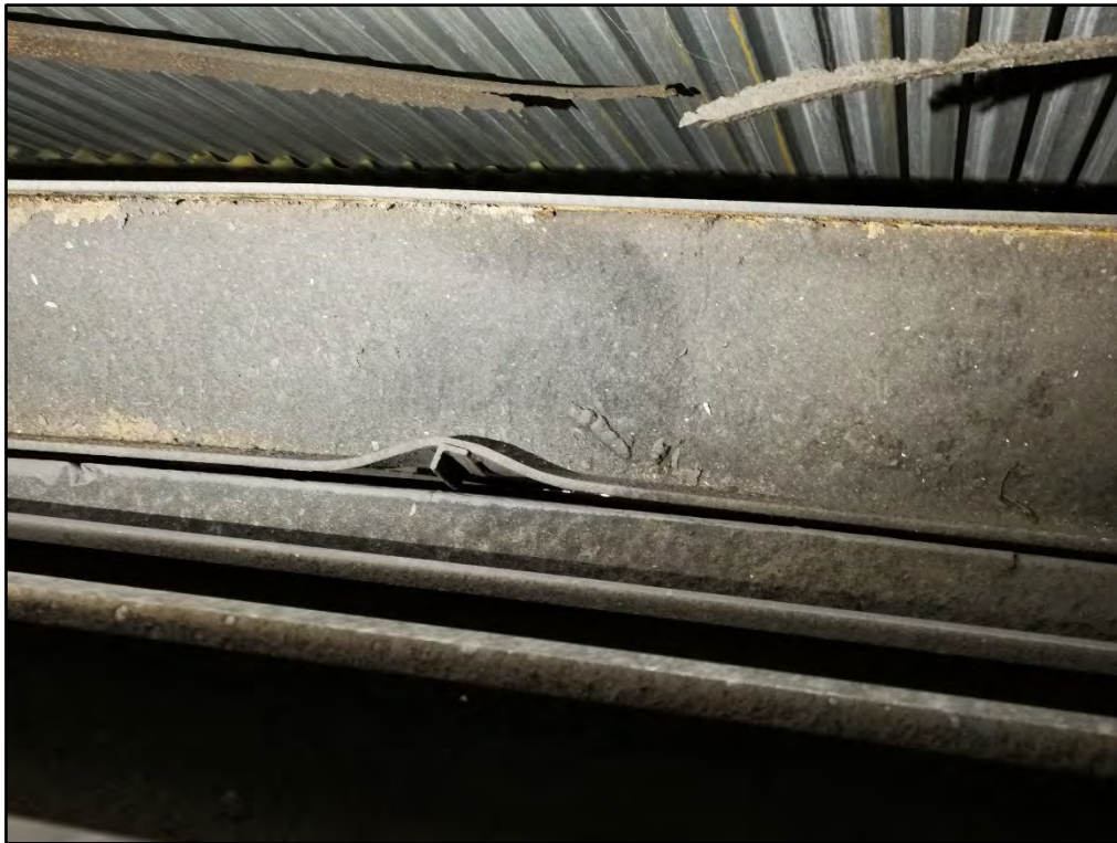
Photograph 150 Damaged PFC Section
