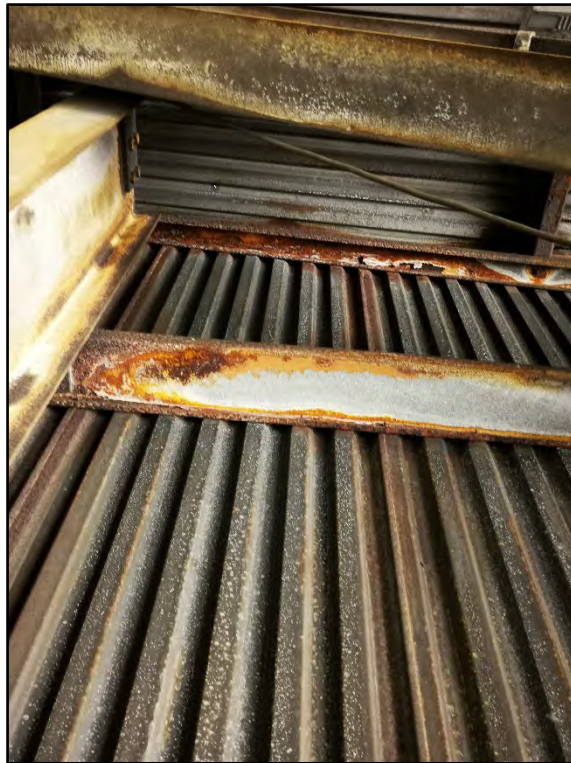
Photograph 162 Delamination of Wall Girts due to Corrosion
