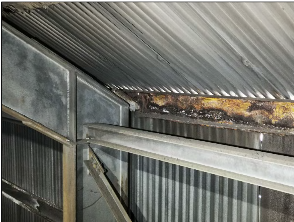
Photograph 34 Delamination of Fascia Purlin due to Corrosion
