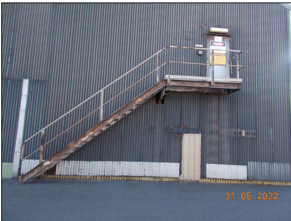
Photograph 49 Stair Stringers Heavily Corroded, wall sheeting patched to lower edge
