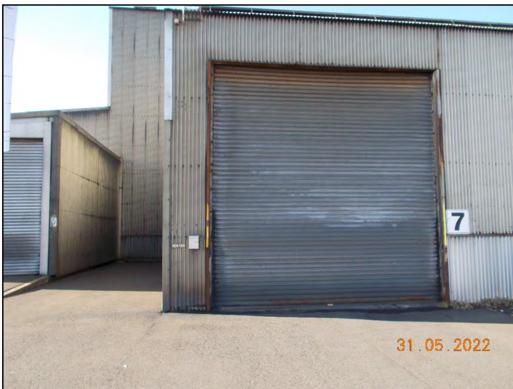
Photograph 47 Heavily Corroded Door Frame
