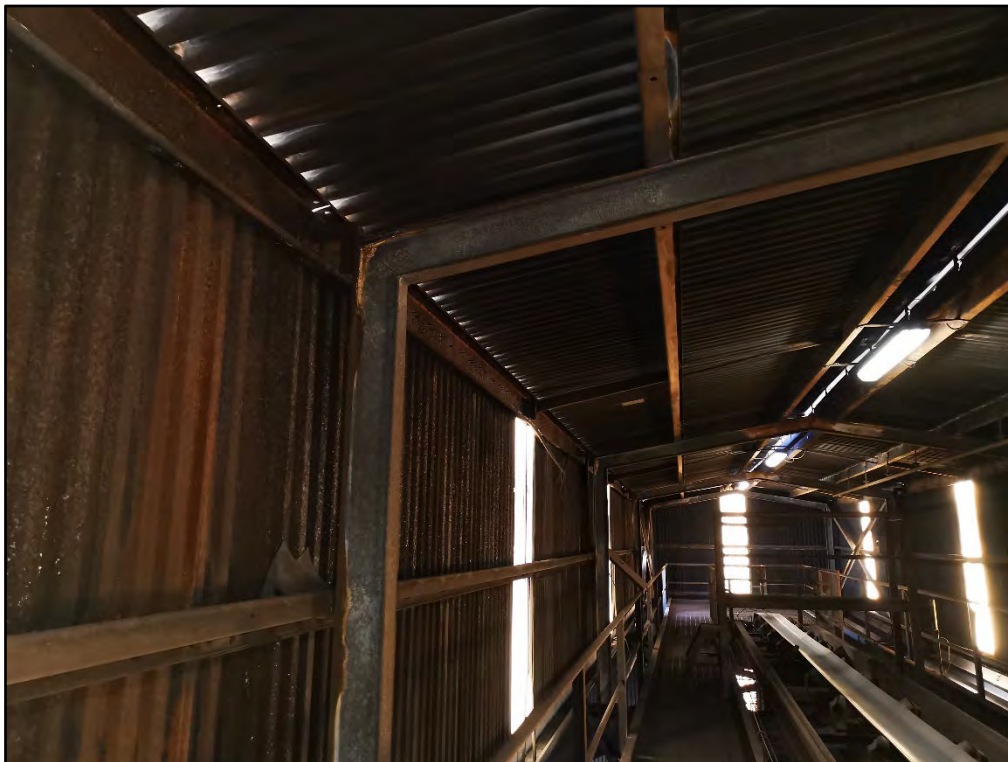
Photograph 169 Surface Corrosion of Steel Members and Damaged Fascia Purlin
