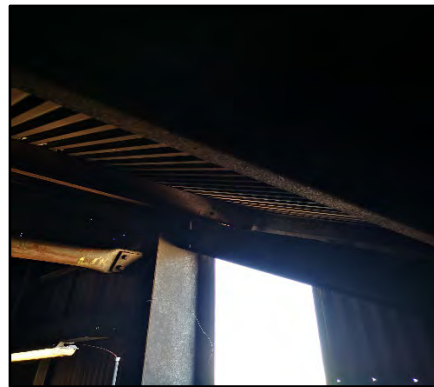
Photograph 43 Shed 6 South Side Sheet Missing on 01 September 2022
