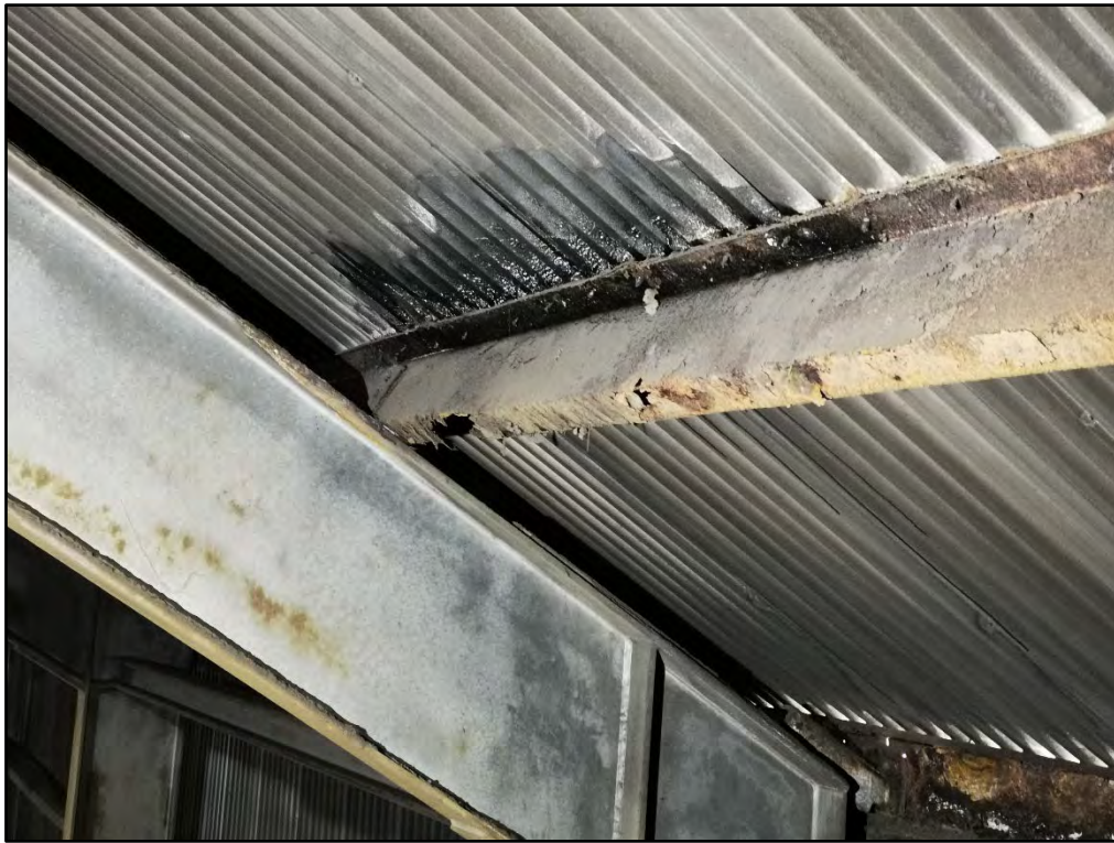
Photograph 35 Deteriorated Purlin due to Corrosion
