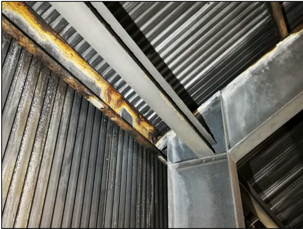
Photograph 112 Corrosion of Fascia Purlin
