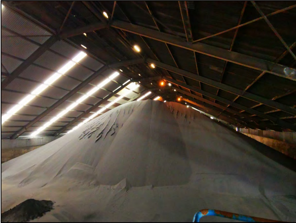
Photograph 134 Product Inside the Shed Restricted the Access
