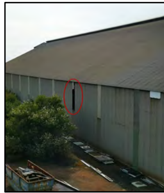
Photograph 60 Shed 7 Eastern Side Sheet Missing on 02 September 2022
