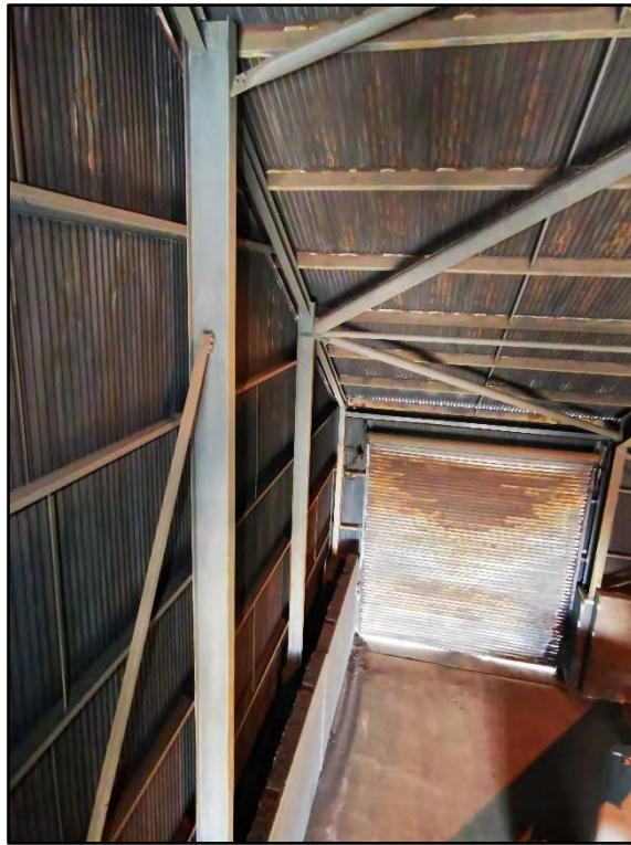
Photograph 108 Surface Corrosion of Purlins, Girts, and Sheeting
