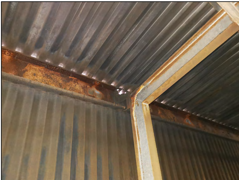
Photograph 167 Heavily Corroded Fascia Purlin on Conveyor and Walkway
