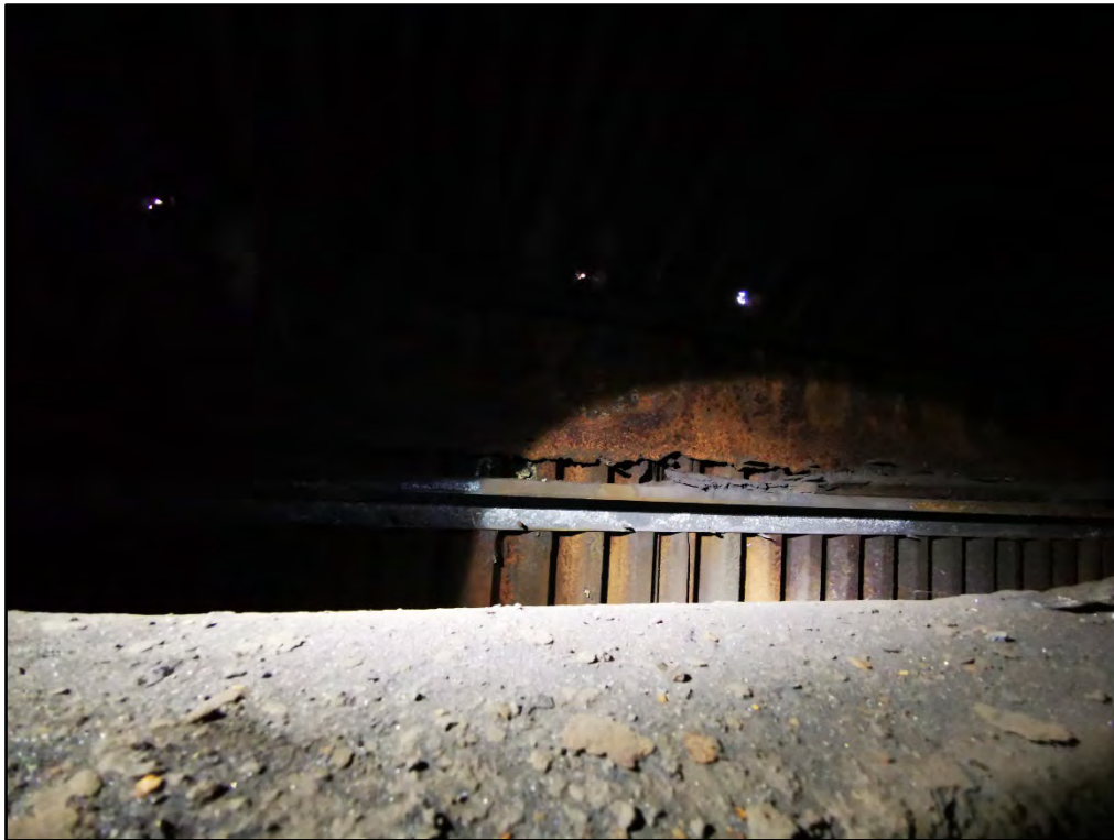
Photograph 25 Deteriorated Fascia Purlin due to Corrosion
