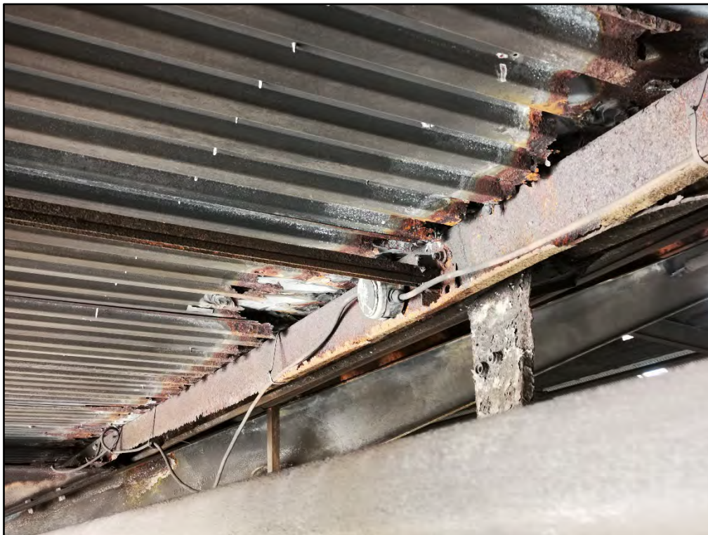
Photograph 147 Deterioration Purlin due to Corrosion
