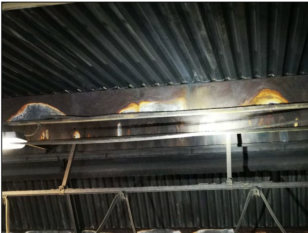
Photograph 79 Surface Corrosion of Purlin with Product Deposit
