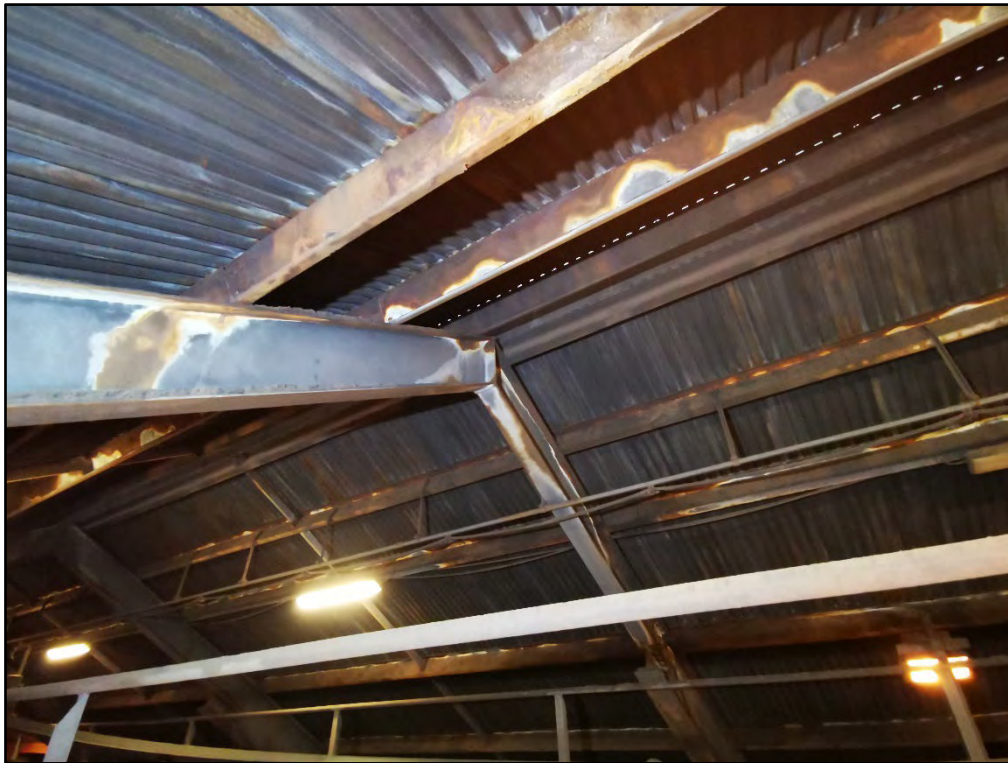
Figure 102 Surface Corrosion of Rafters, Purlins and Roof Sheeting
