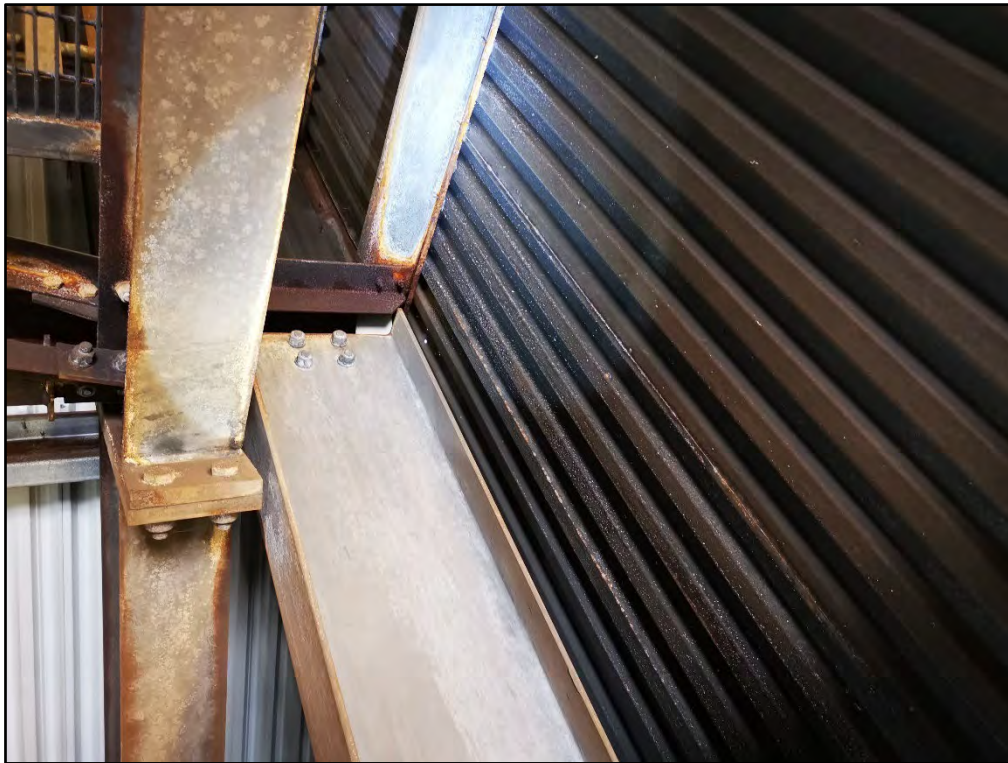
Photograph 160 Heavily Corroded EA Section
