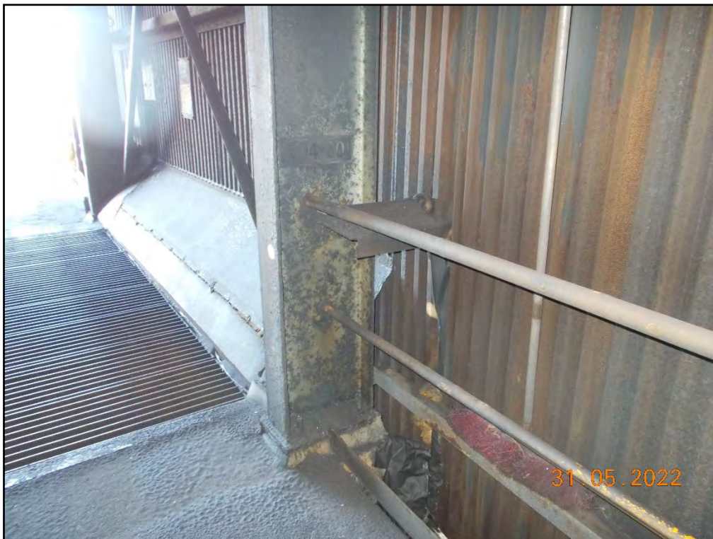
Photograph 64 Corrosion of Wall Sheeting
