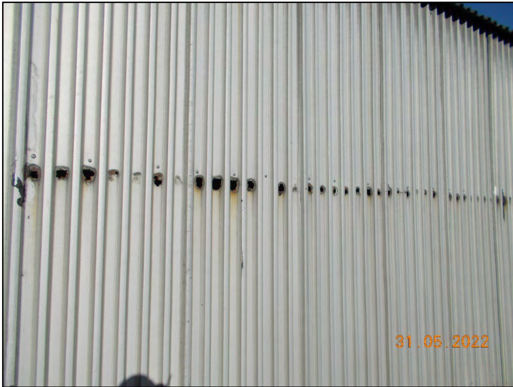
Photograph 124 Deterioration Due to Corrosion
