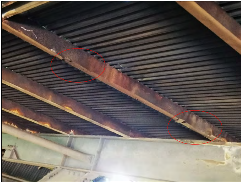
Photograph 21 Damaged Purlin and Surface Corrosion of Purlins
