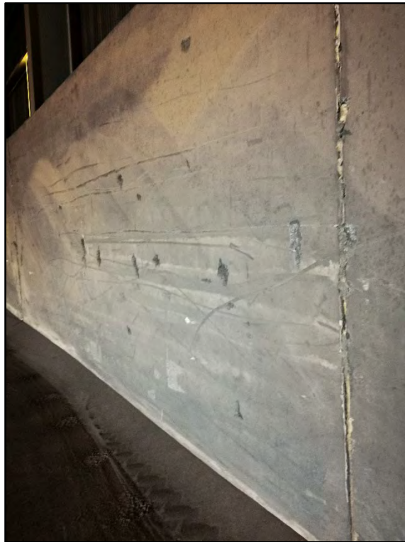
Photograph 118 Minor Impact Damages Due to Loader
