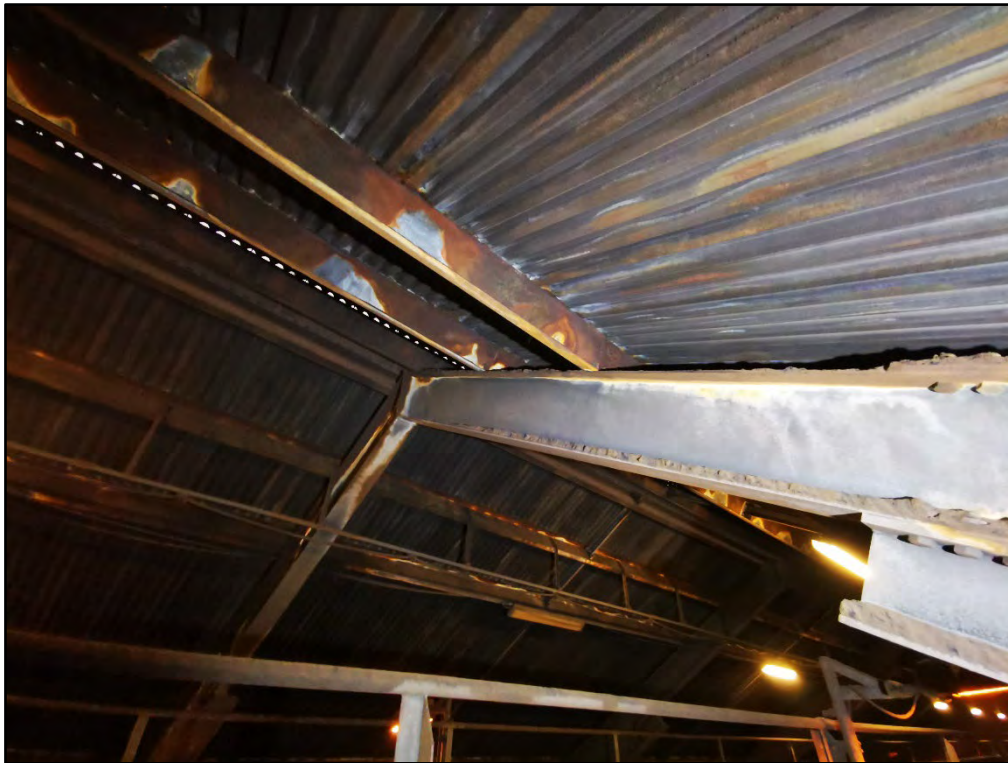
Photograph 100 Surface Corrosion of Rafters, Purlin and Roof Sheeting with Product Deposit
