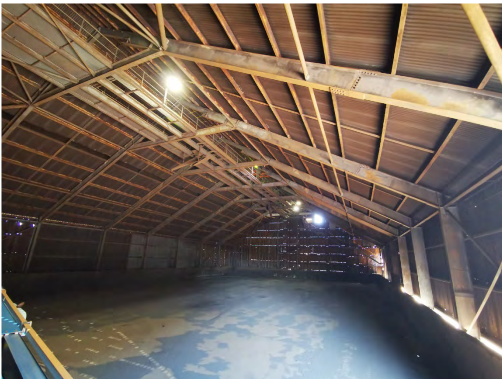
Photograph 38 Surface Corrosion of Roof Sheetting
