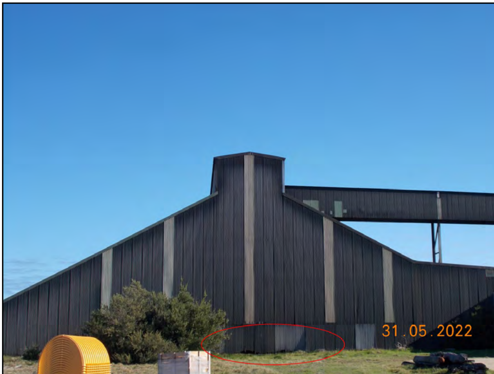
Photograph 131 Deterioration at the Bottom of Wall Sheeting
