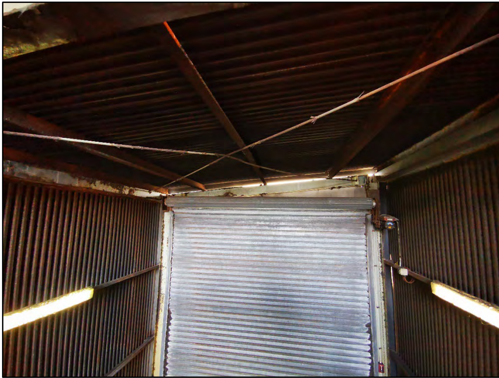
Photograph 16 Damage to Purlin and Bracing due to Impact
