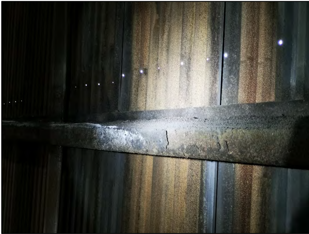
Photograph 31 Heavily Corroded Girt
