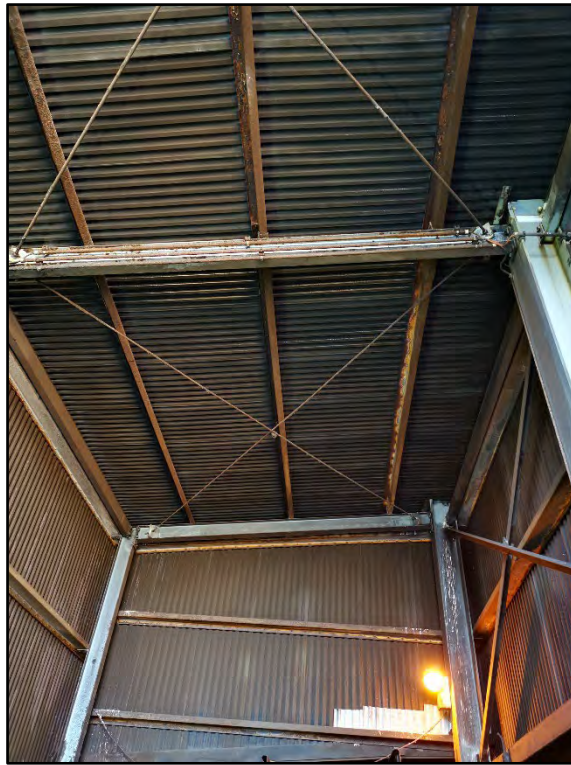
Photograph 14 Surface Corrosion of Purlins, Columns and Rafters
