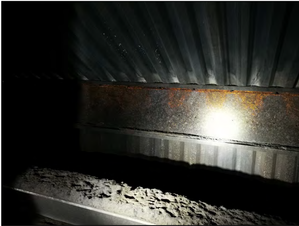
Photograph 80 Corrosion of Fascia Purlin and Product Deposit
