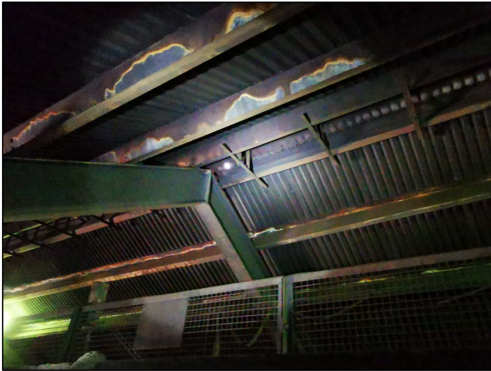
Photograph 23 Surface Corrosion of Purlins and Rafters
