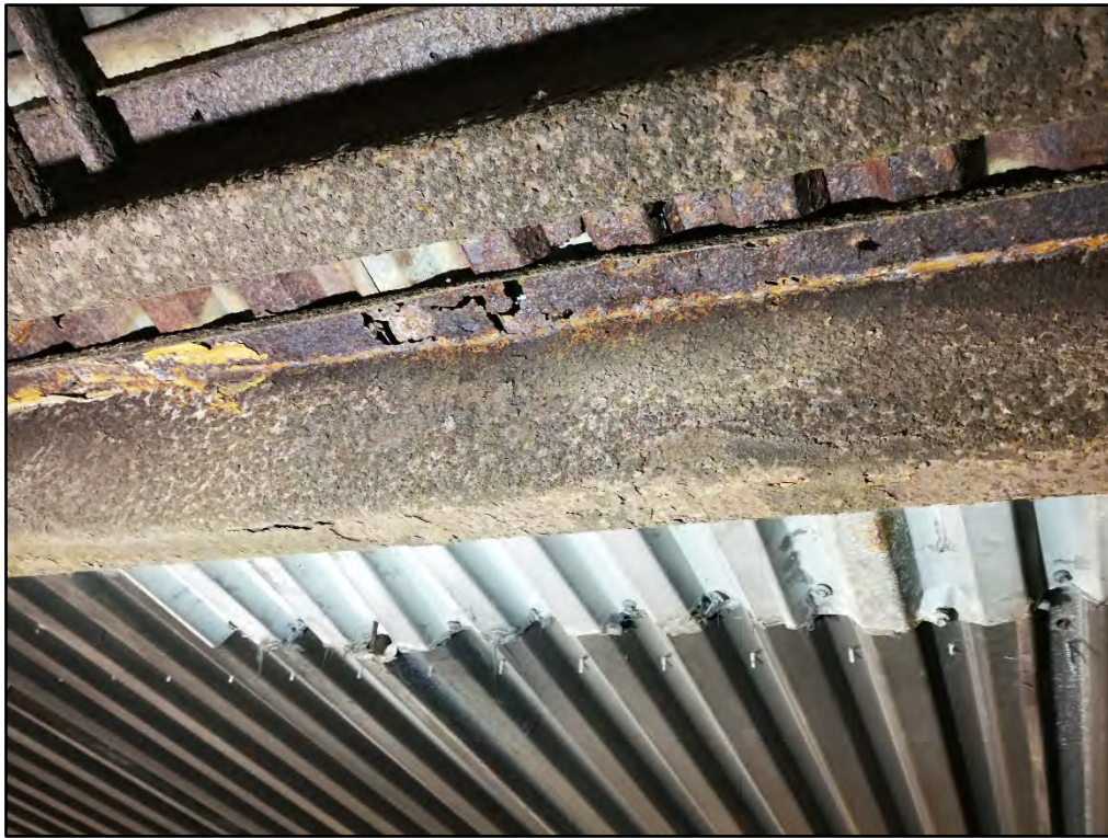
Photograph 148 Heavily Corroded Purlin
