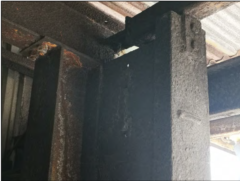
Photograph 146 Heavily Corroded Steel Members
