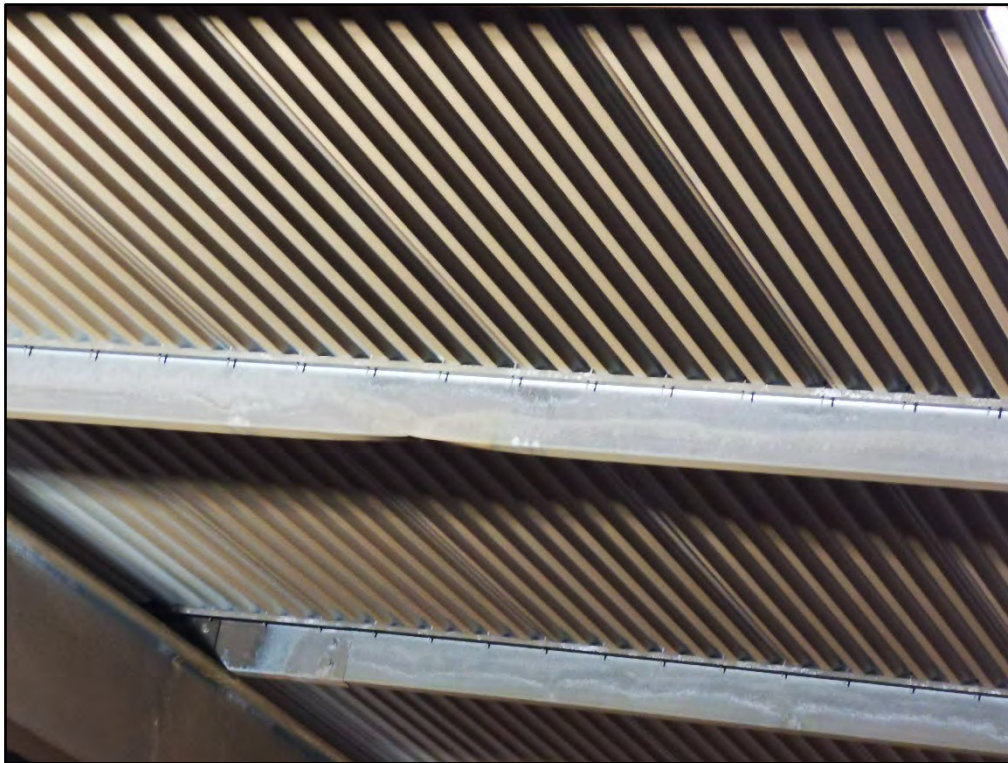
Photograph 154 Damaged Purlin due to Impact in South Side
