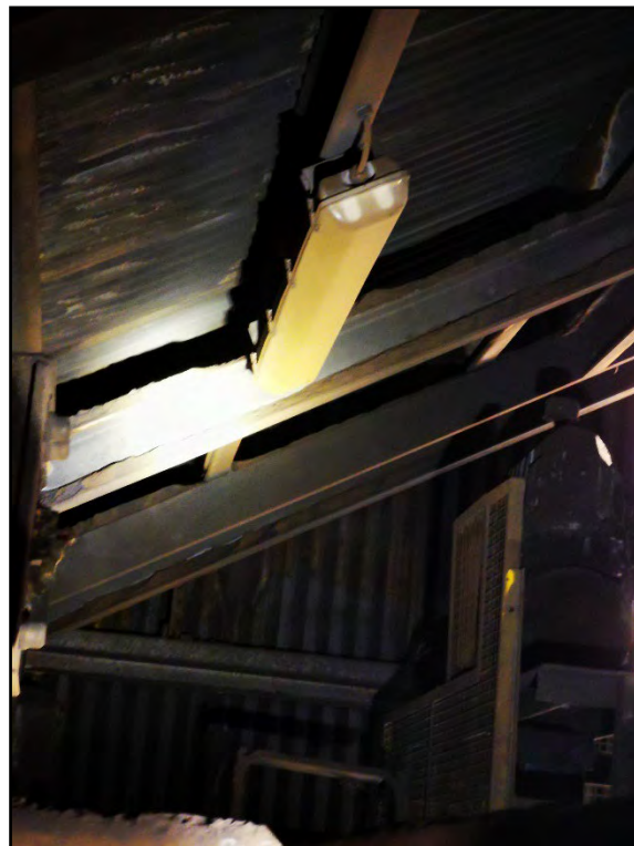
Photograph 77 Surface Corrosion of Purlin and Roof Sheeting and Product Deposit on Flanges of UB Section
