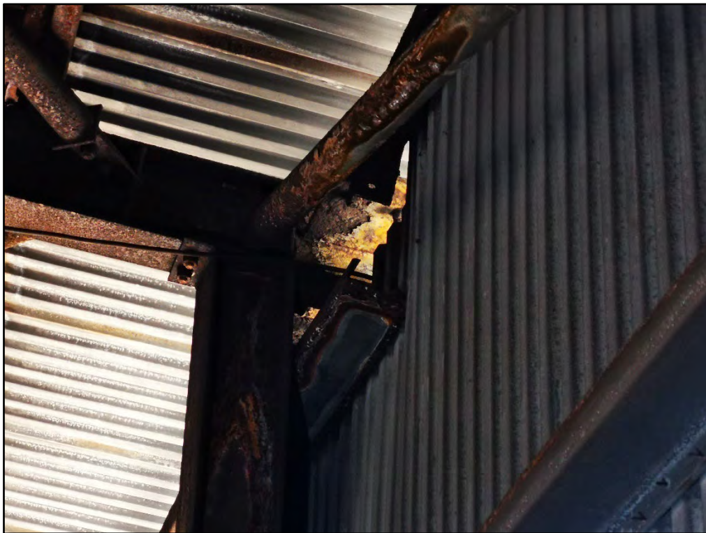
Figure 149 Heavily Corroded Steel Members
