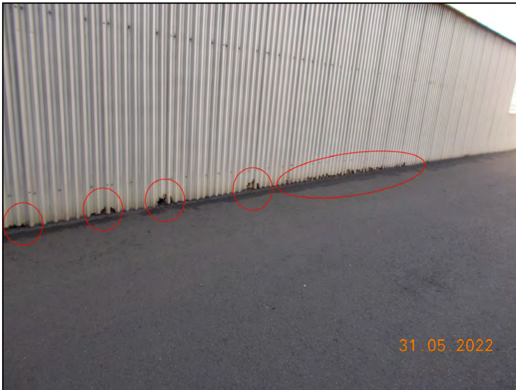
Photograph 123 Corrosion Deterioration Observed at the Bottom
