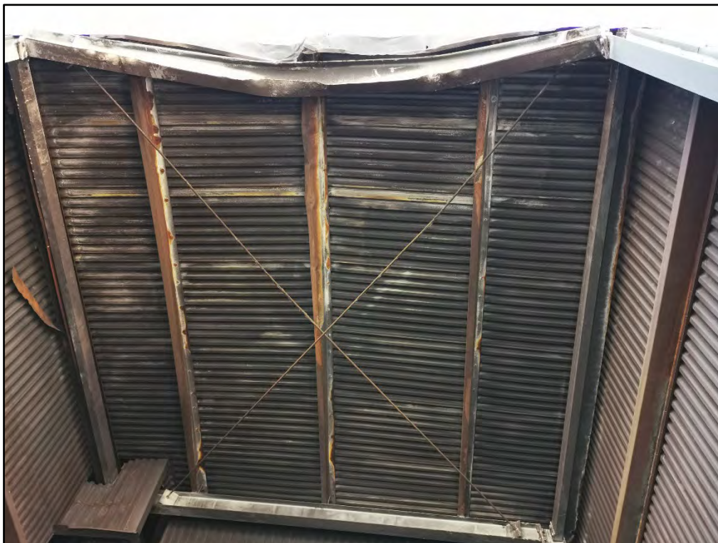
Photograph 68 Impact Damage Due to Vehicle
