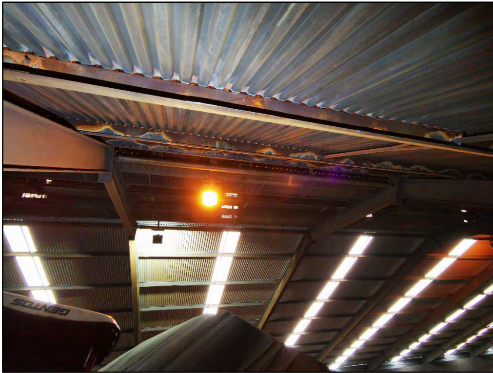
Photograph 144 Surface Corrosion of Purlins and New Purlins and Roof Sheeting in Southern Side
