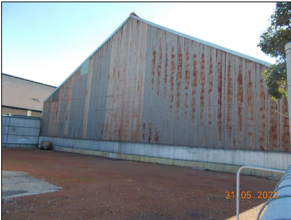
Photograph 7 Corrosion on Wall Sheeting
