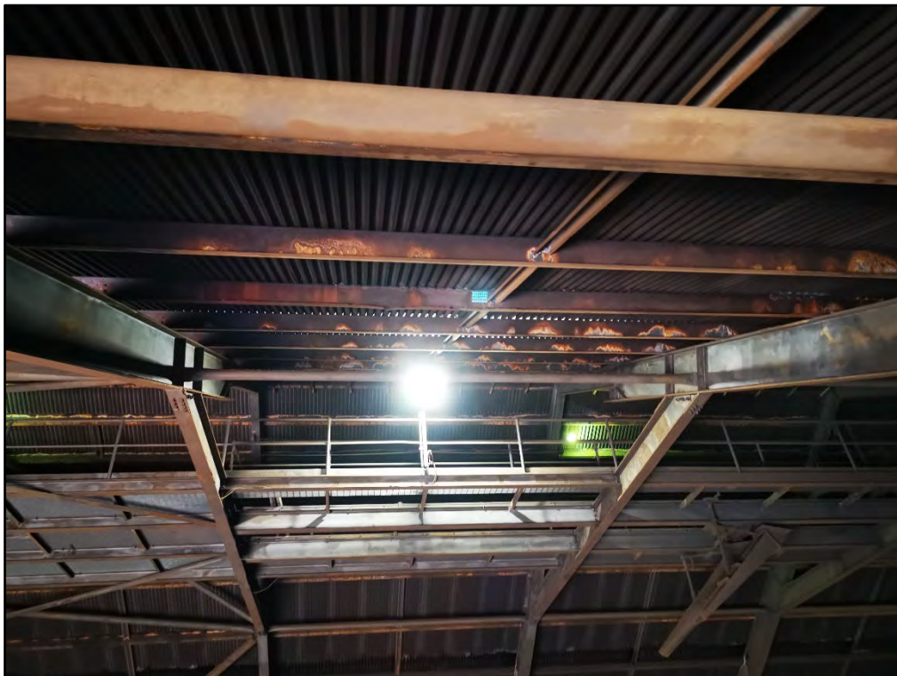
Photograph 20 Surface Corrosion of Purlins
