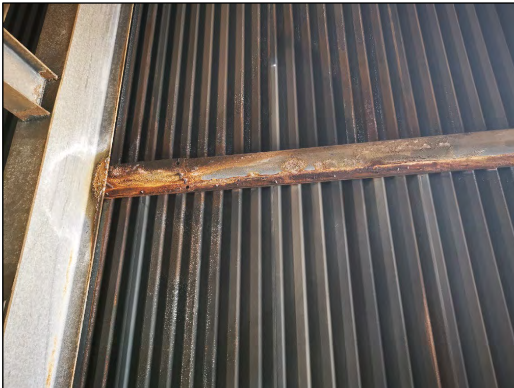
Photograph 161 Heavily Corroded Wall Girt
