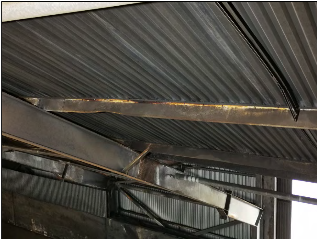
Photograph 142 Damaged Purlin due to Impact
