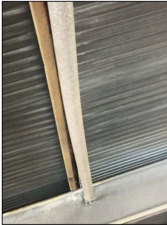
Photograph 164 Deformed CHS Section
