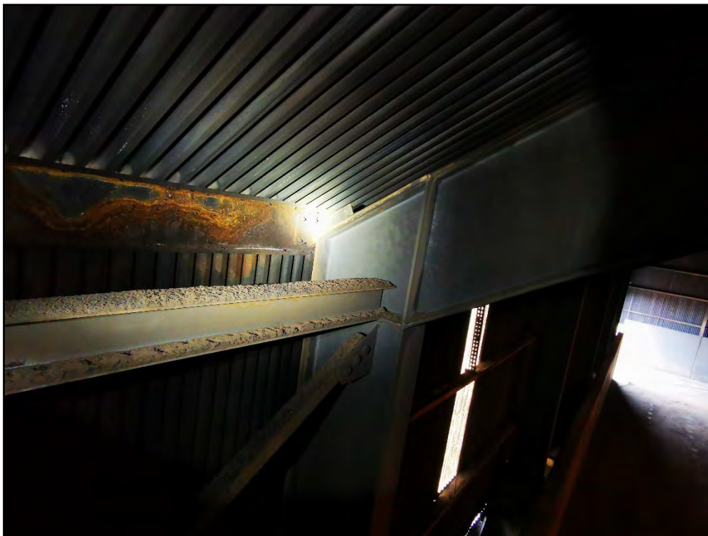
Photograph 87 Corrosion of Fascia Purlin and Product Deposit
