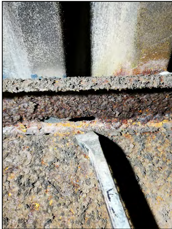
Photograph 94 Sectional Loss of Purlin Due to Corrosion
