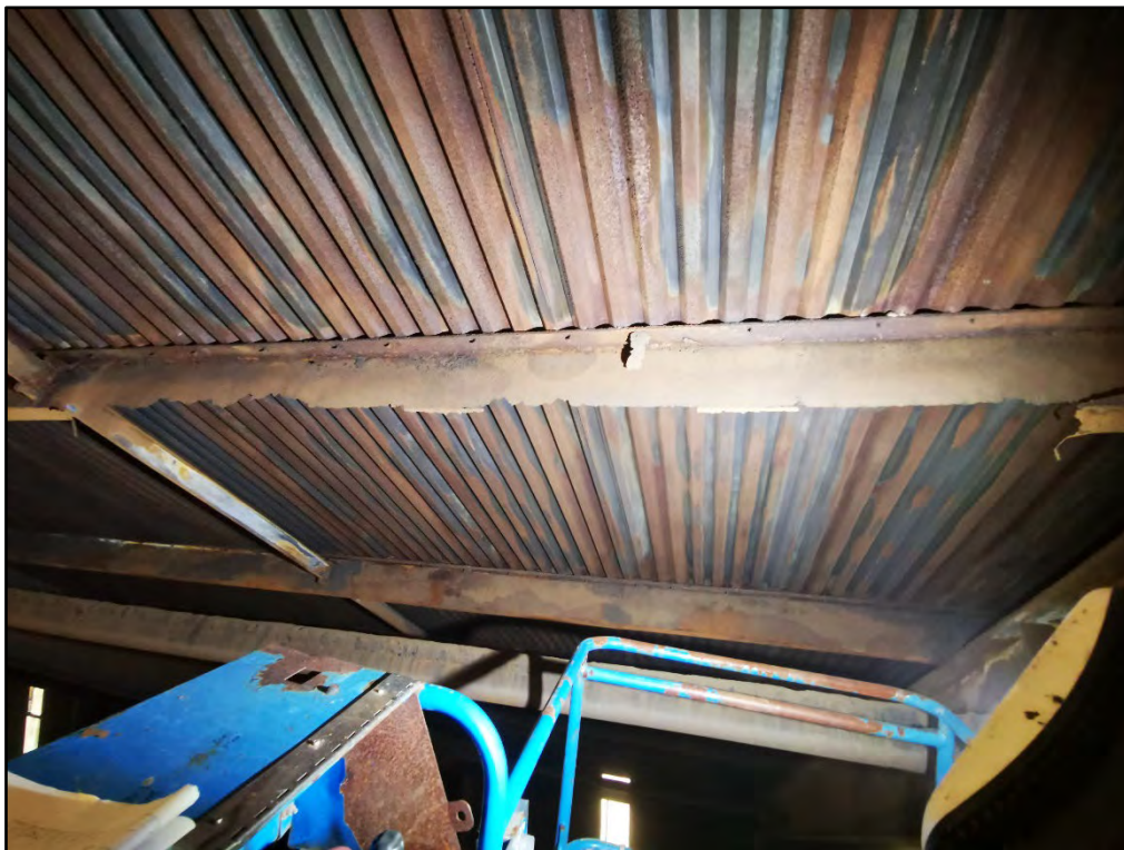
Photograph 95 Sectional Loss of Purlin Due to Corrosion and Roof Sheetting
