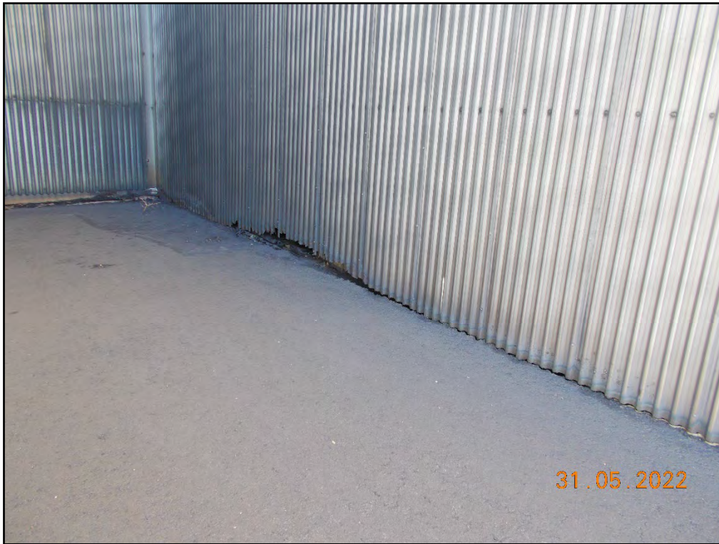
Photograph 52 Damage Observed Due to Corrosion
