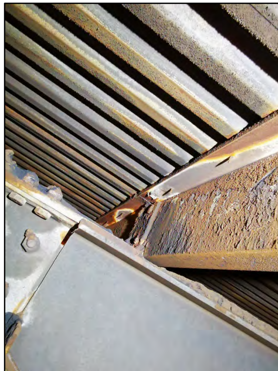
Photograph 105 Surface Corrosion of Bolts, Rafter and Purlin Due to Product Deposit
