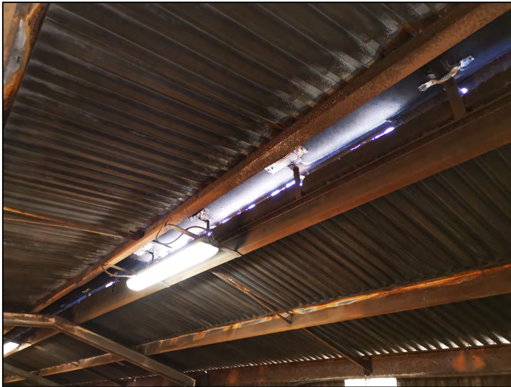
Photograph 166 Heavily Corroded Purlins on Conveyor and Walkway
