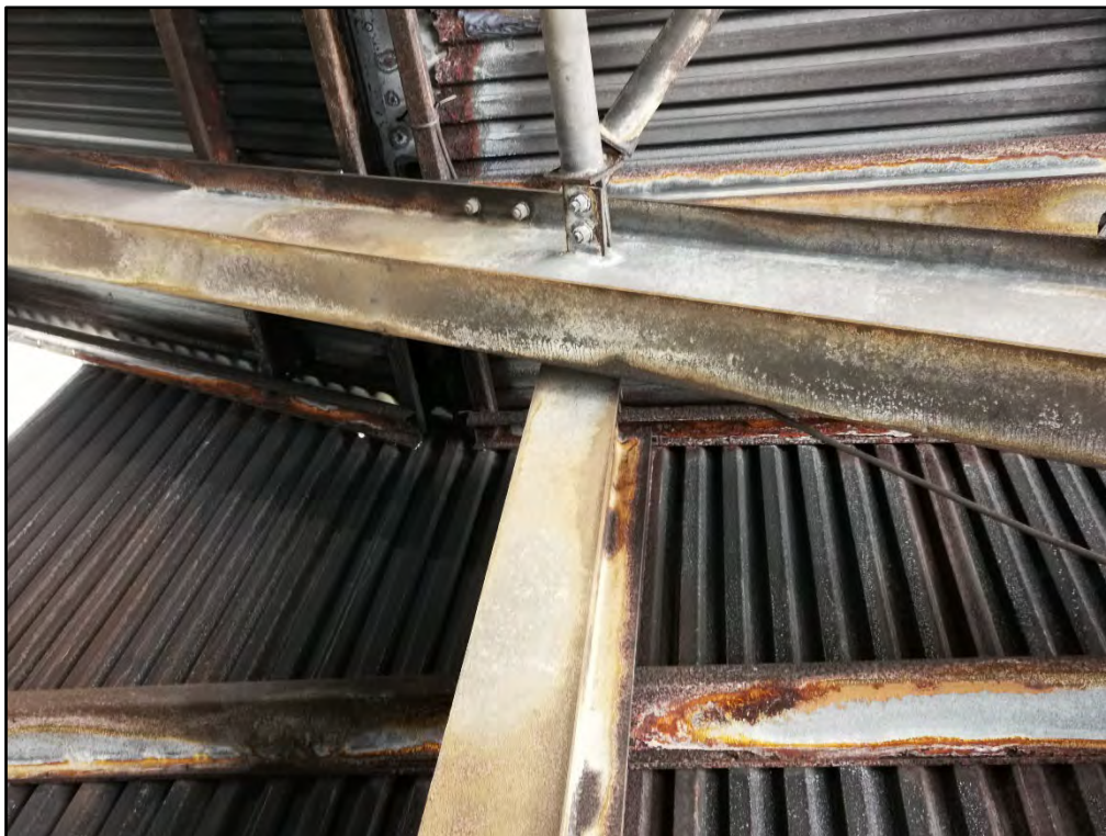
Photograph 163 Delamination of Wall Girts due to Corrosion
