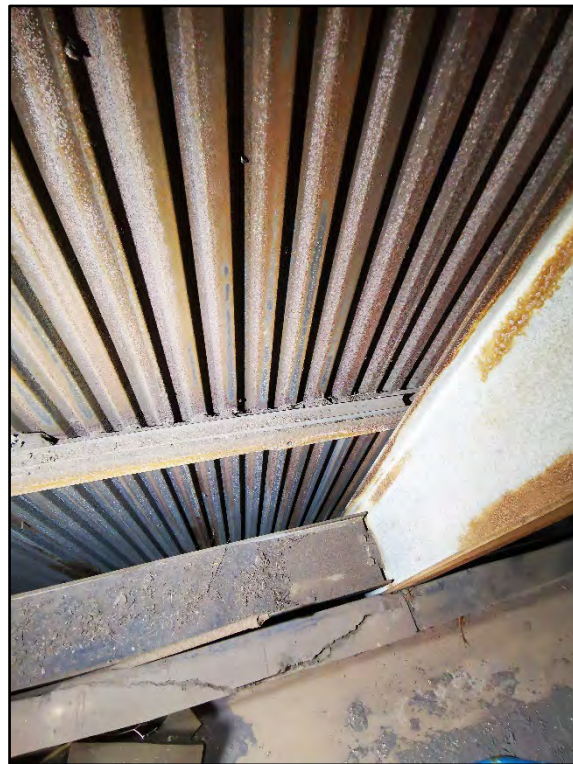
Photograph 145 Cracked Concrete Wall
