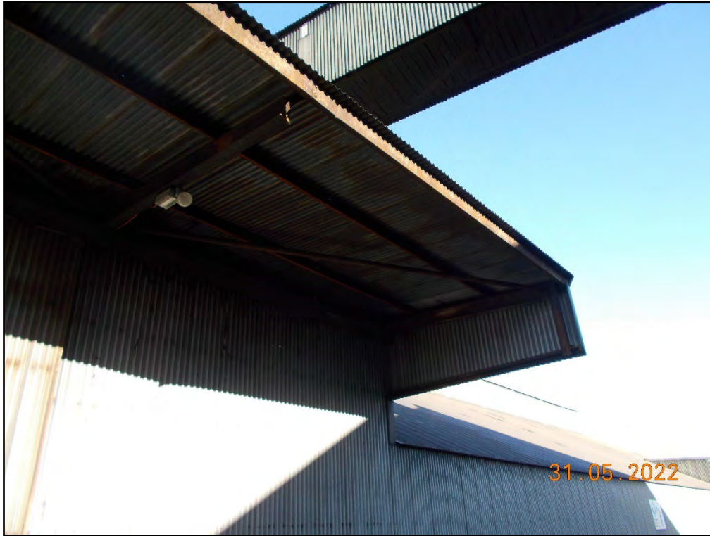
Photograph 122 Corrosion of Rafters and Purlins.
