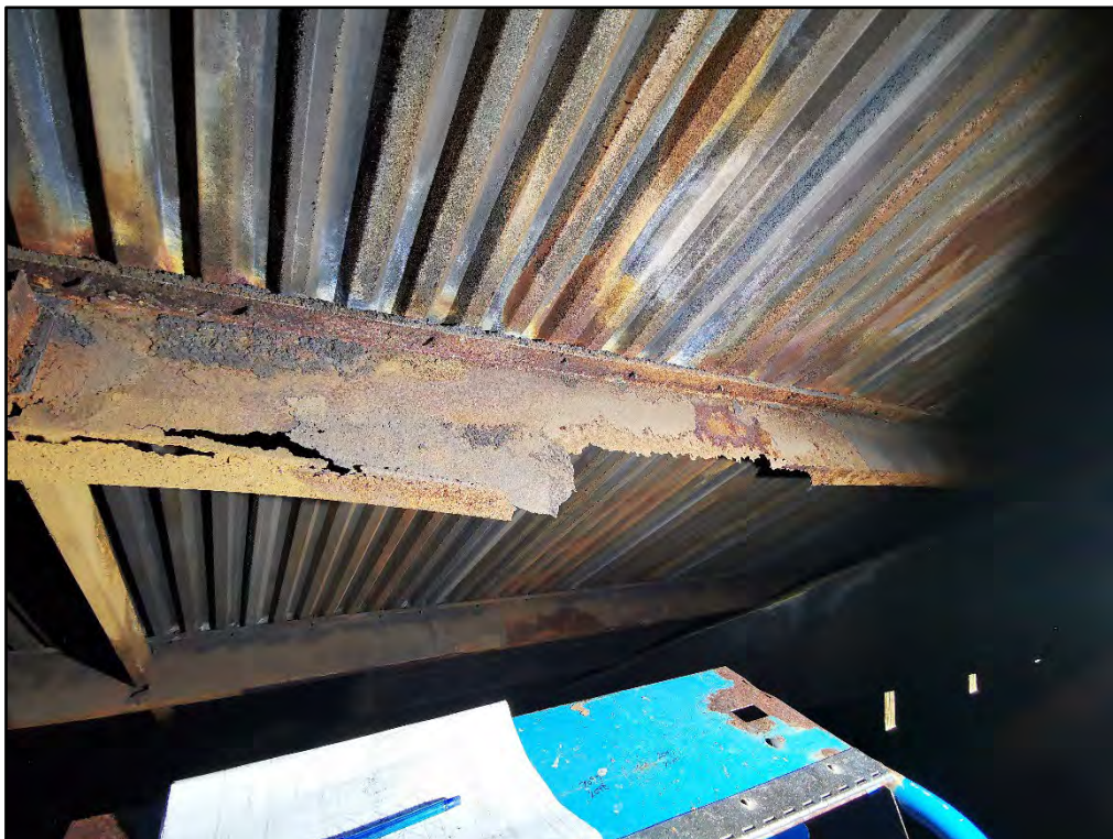
Photograph 97 Sectional Loss of Purlin and Corrosion of Roof Sheeting
