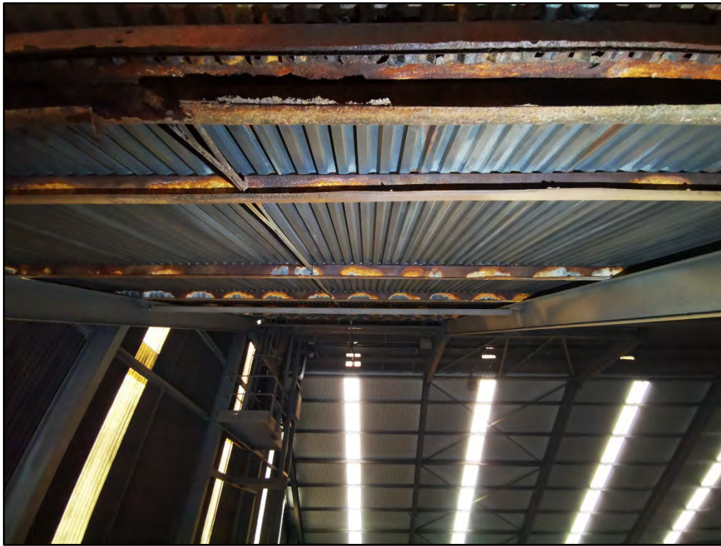
Photograph 140 Deterioration to Purlin and New Purlins and Roof Sheetting on South Side
