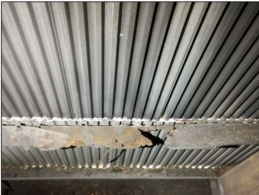
Photograph 91 Complete Failure of Wall Girt
