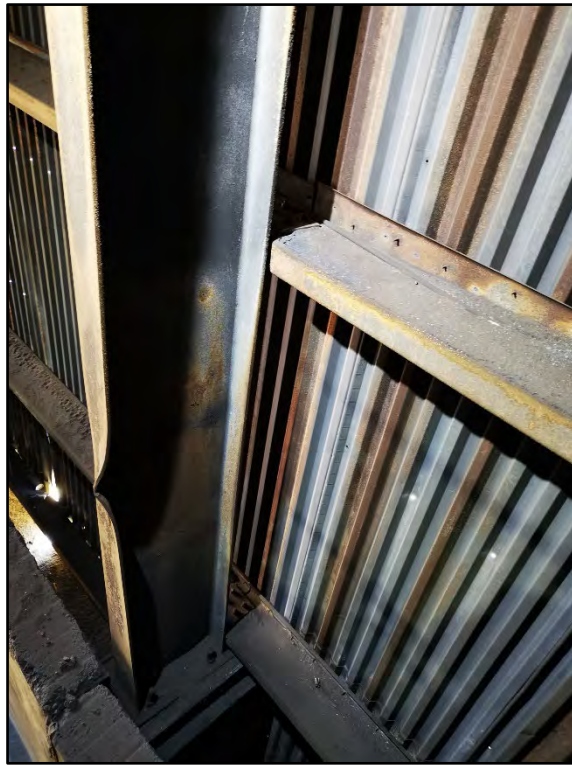
Photograph 37 Impact Damage of Column
