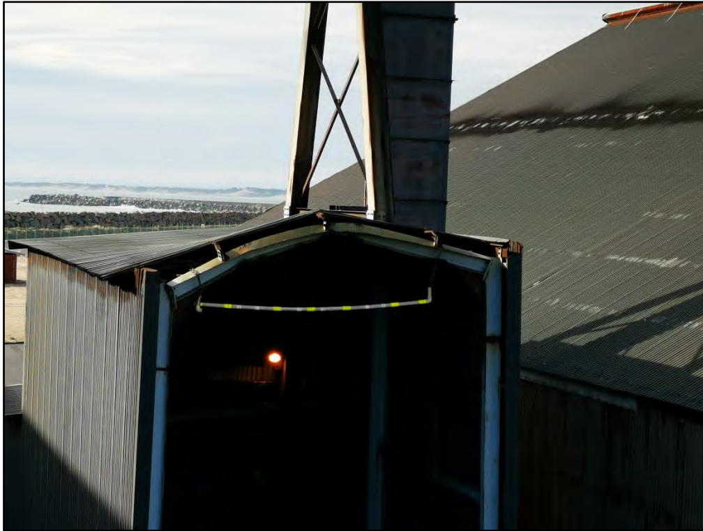
Photograph 12 Impact Damage on Rafter in Unloading Bay
