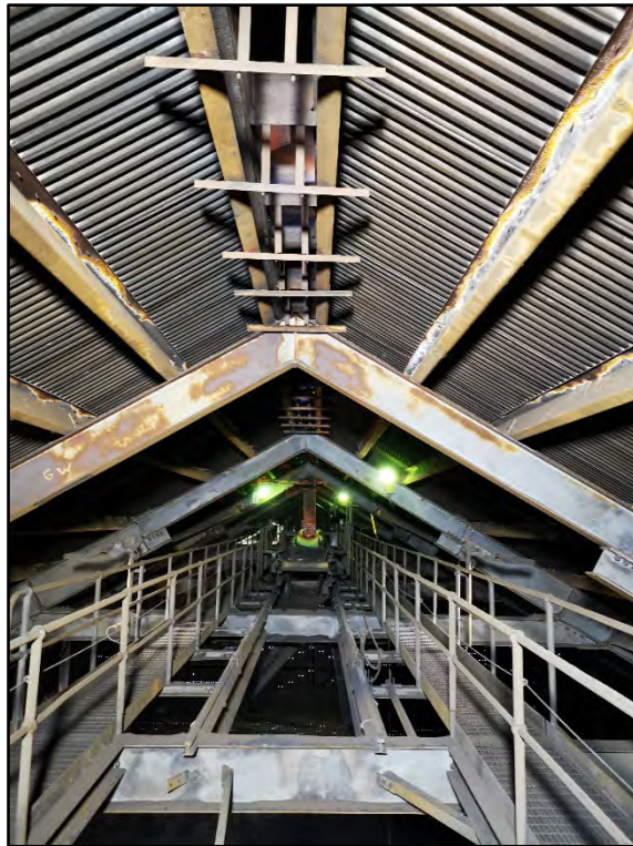
Photograph 39 Surface Corrosion of Purlins and Rafters on Walkway and Conveyor
