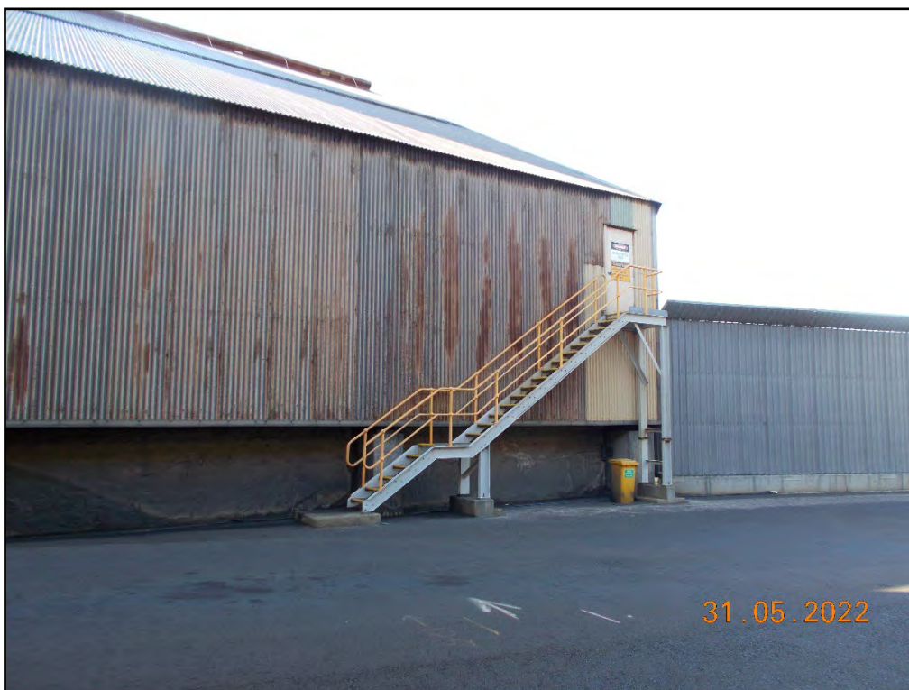
Photograph 5 Corrosion on Wall Sheeting
