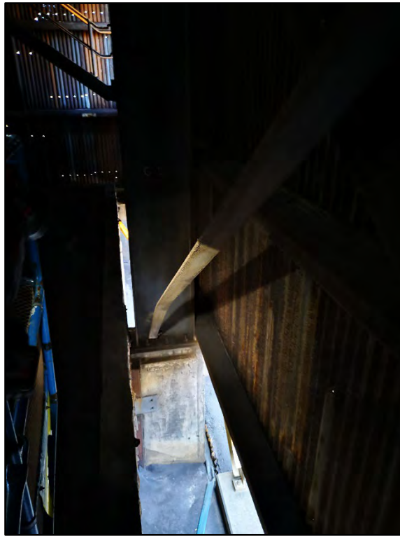
Photograph 29 Bent Cross Brace
