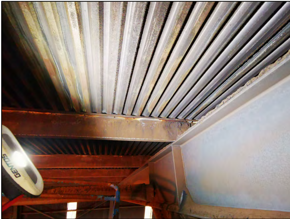
Photograph 106 Surface Corrosion of Bolts, Rafter and Purlin Due to Product Deposit
