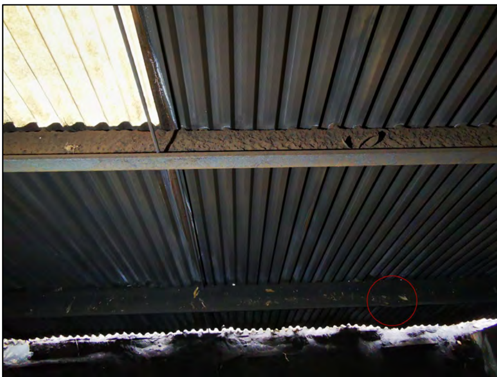
Photograph 101 Damage to Girt Due to Product Deposit
