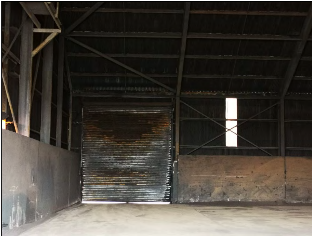
Photograph 74 Door Frame Showing Signs of Corrosion
