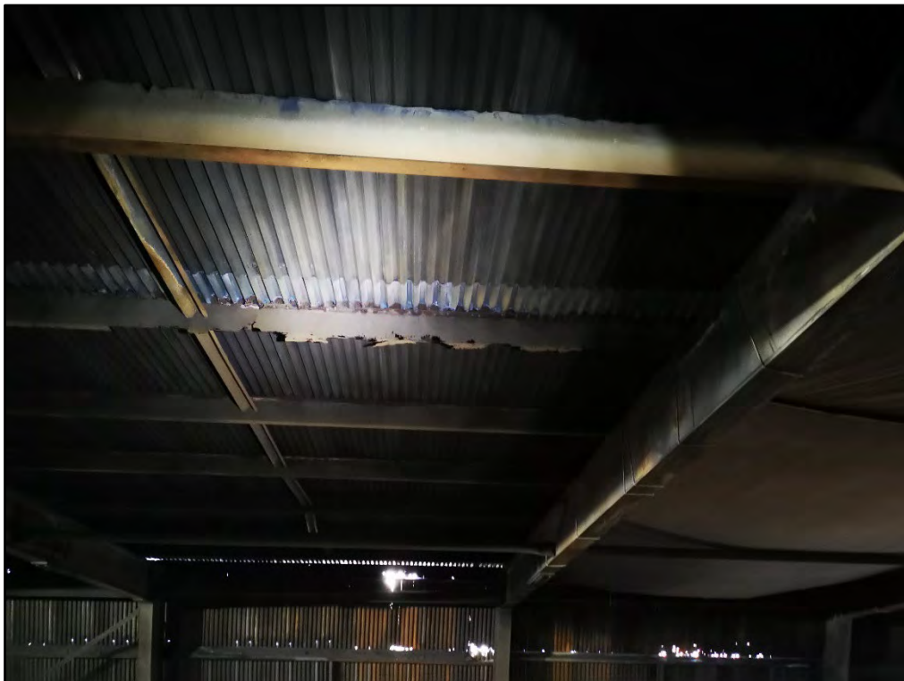
Photograph 26 Deteriorated Purlin due to Corrosion
