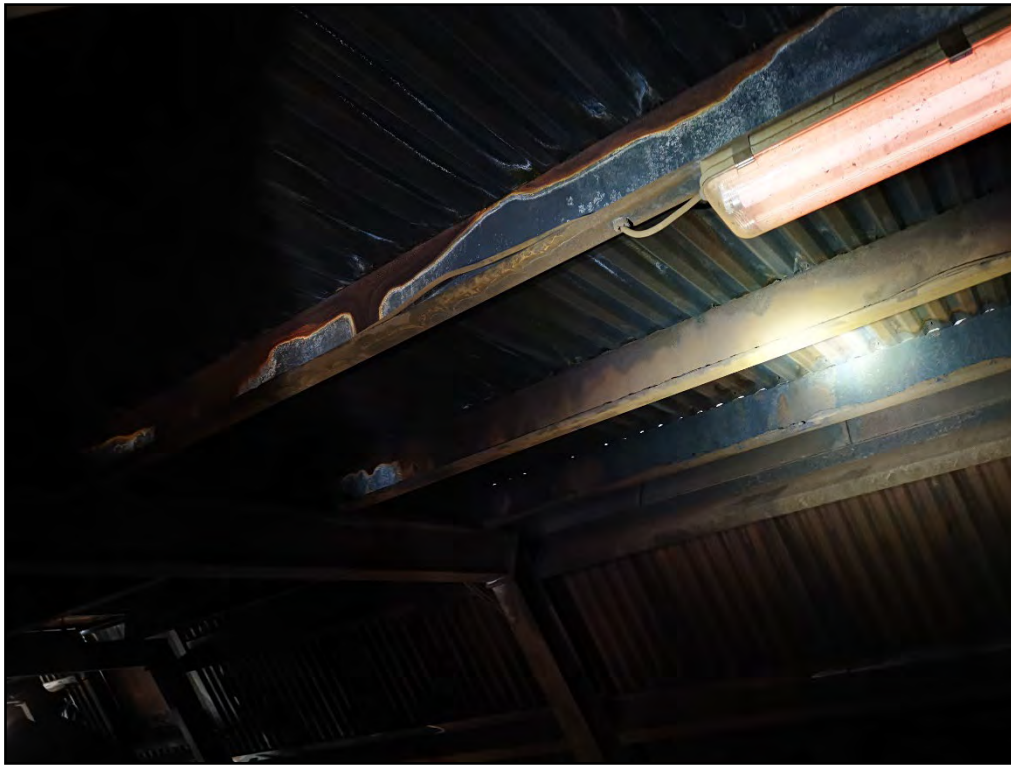
Photograph 76 Surface Corrosion of Purlins
