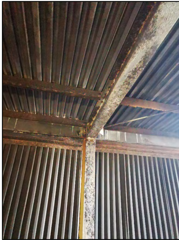
Photograph 69 Surface Corrosion of Columns, Rafter, and Purlins
