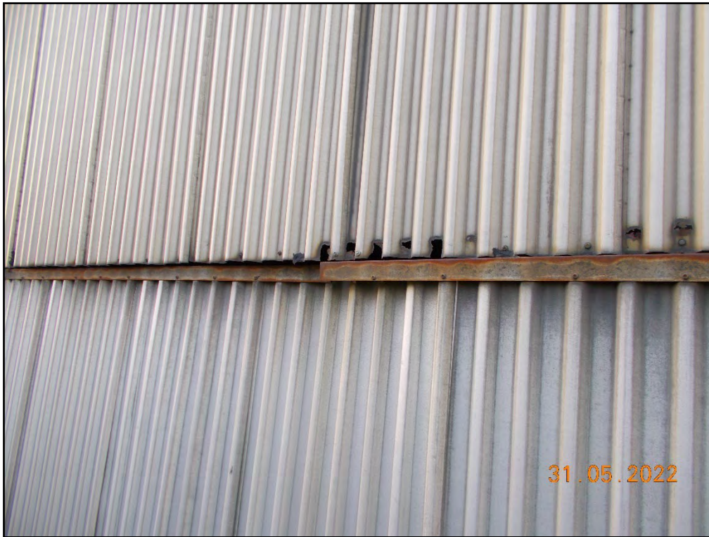
Photograph 48 Surface Corrosion of Steel Member and Wall Sheeting
