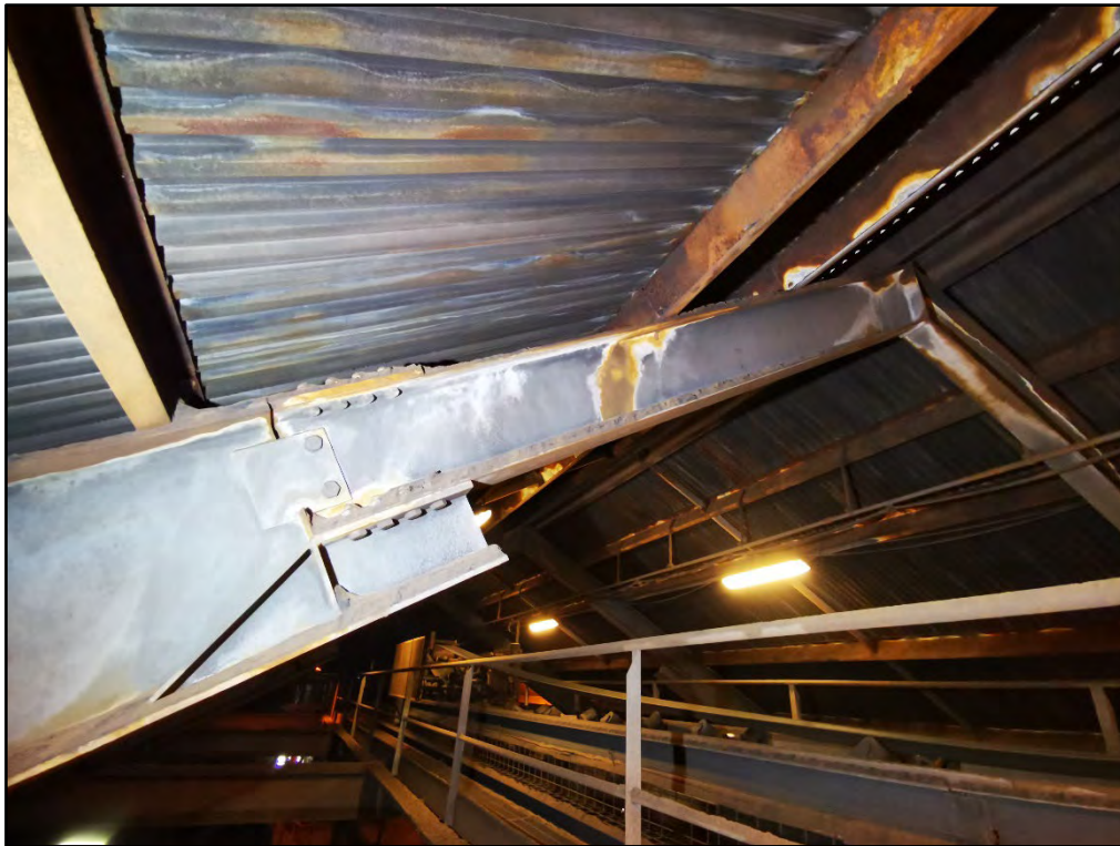
Photograph 96 Surface Corrosion of Purlins and Rafters
