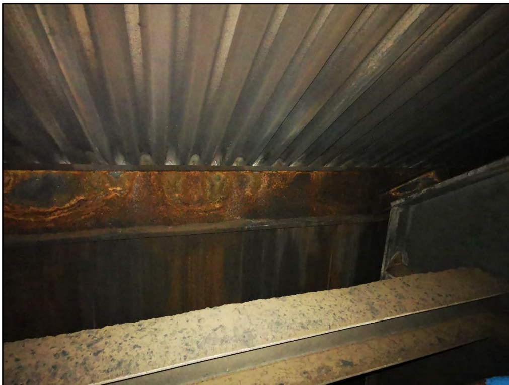
Photograph 83 Corrosion of Fascia Purlin and Product Deposit on UB Section
