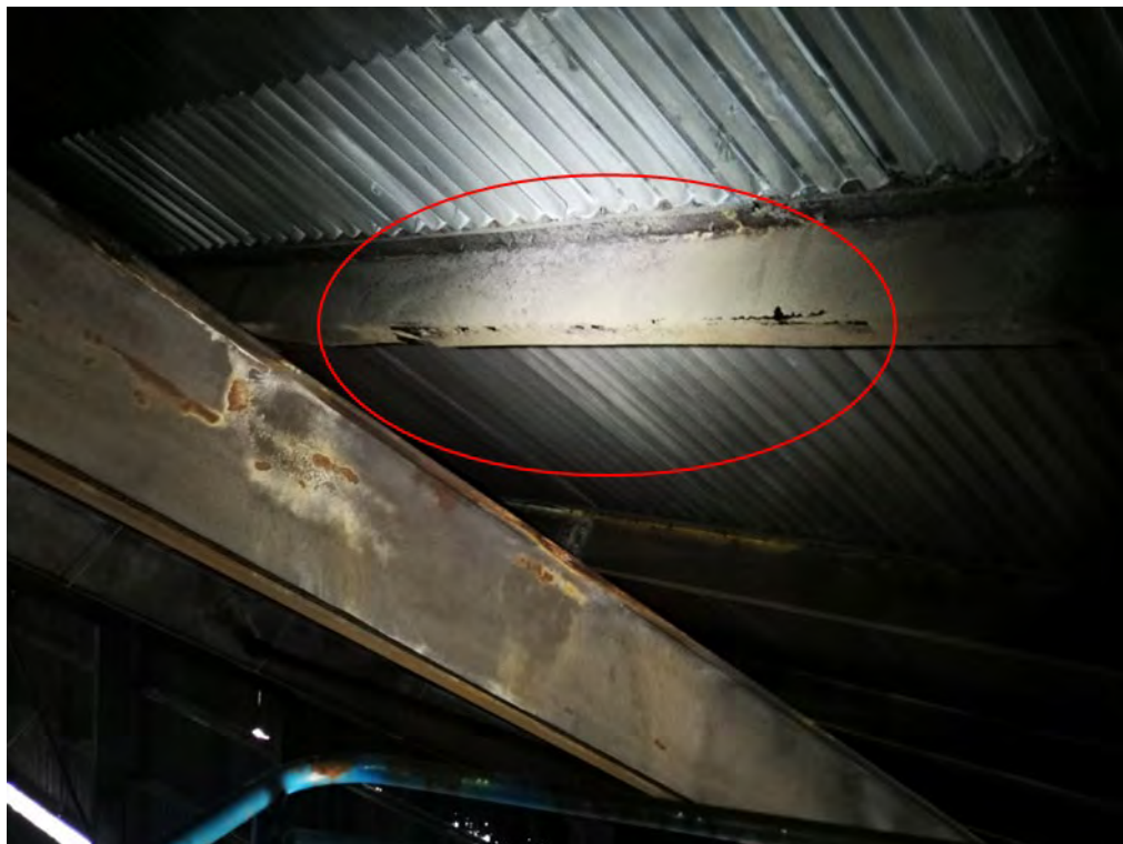
Photograph 22 Deteriorated Purlin due to Corrosion
