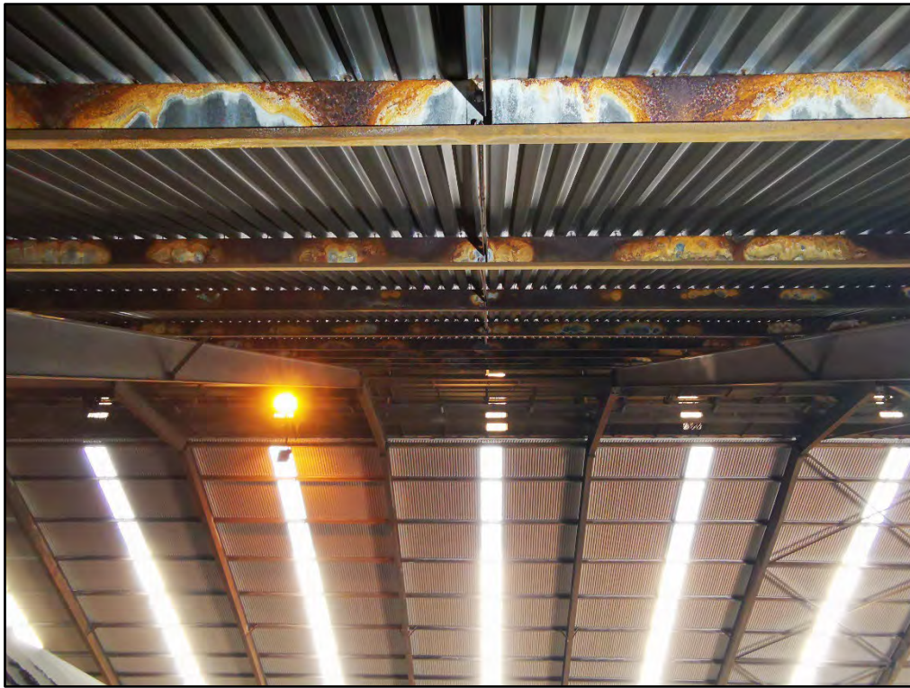
Photograph 152 Surface Corrosion of Purlins
