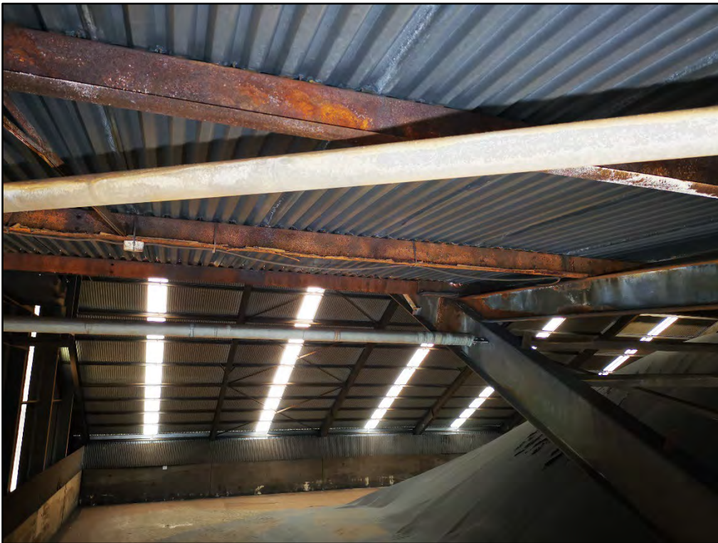
Photograph 135 Deteriorated Purlin due to Corrosion
