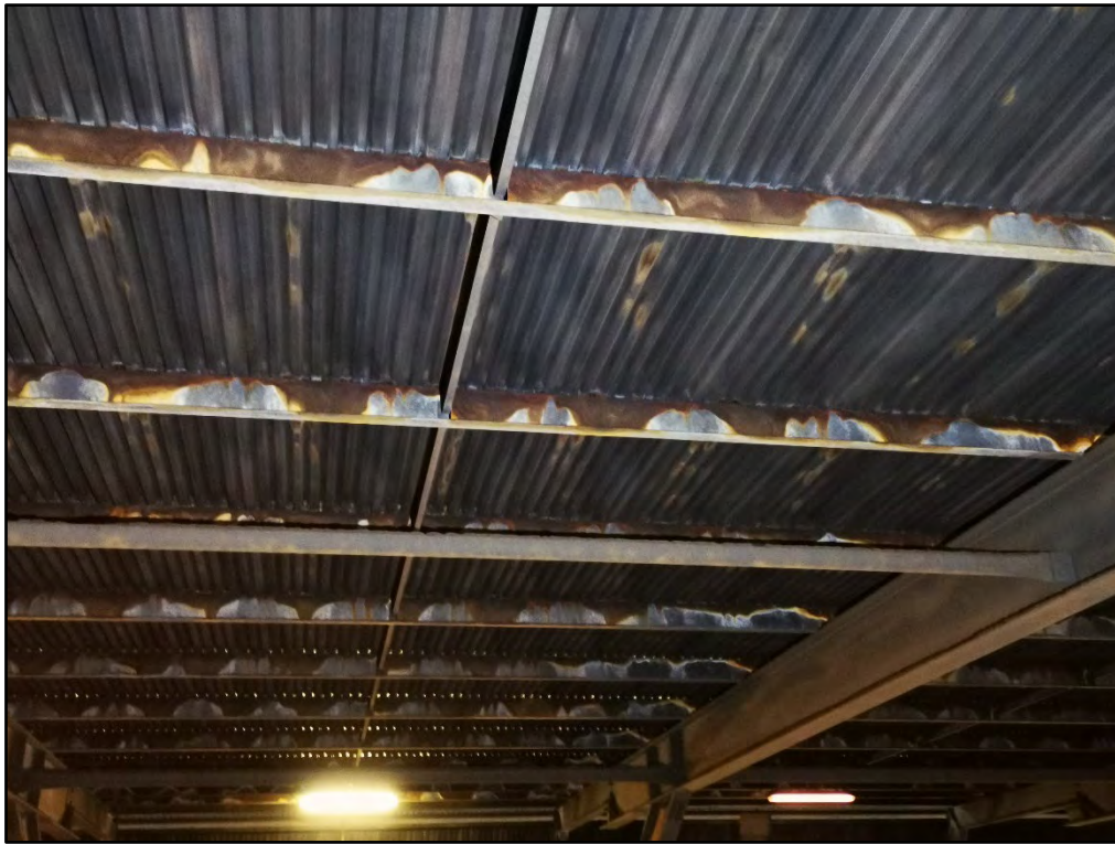
Photograph 104 Surface Corrosion of Purlins and Roof Sheeting
