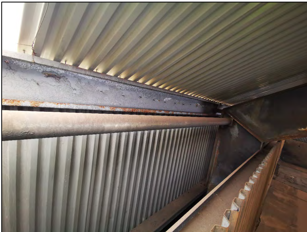
Photograph 157 Surface Corrosion of Fascia Purlin
