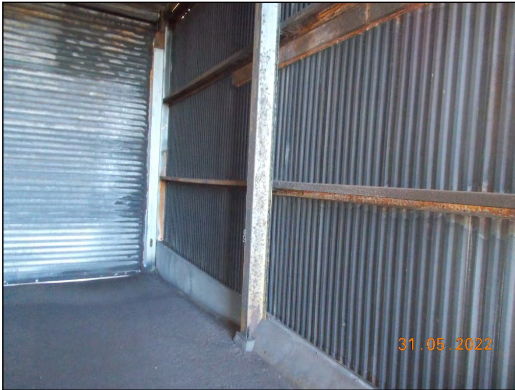
Photograph 65 Heavy Corrosion of Girts
