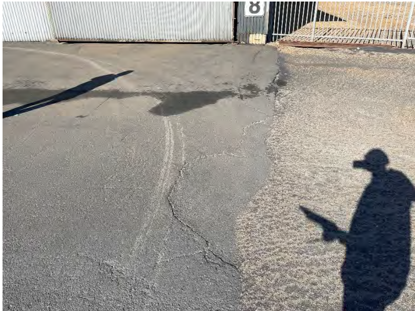
Photo 20: Damage on road edge and standing water in front of shed 8
