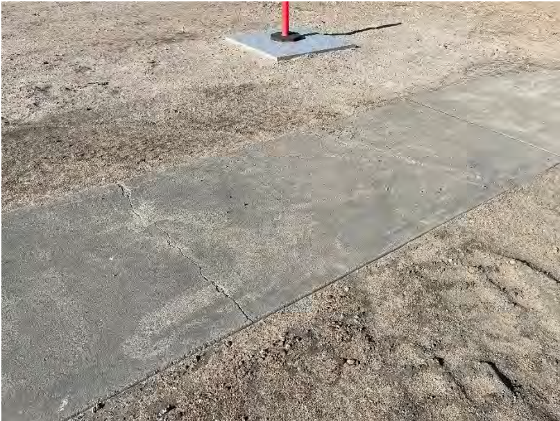
Photo 11: Cracks through the concrete path
