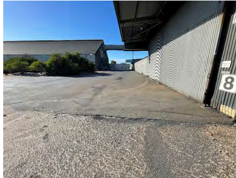
Photo 23: Require gravel top-up on road edge
