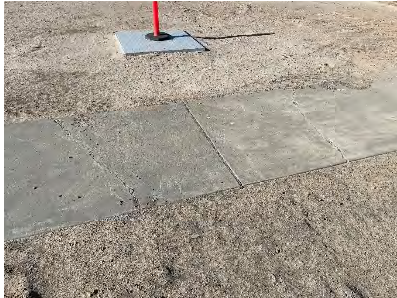
Photo 12: Cracks through the concrete path
