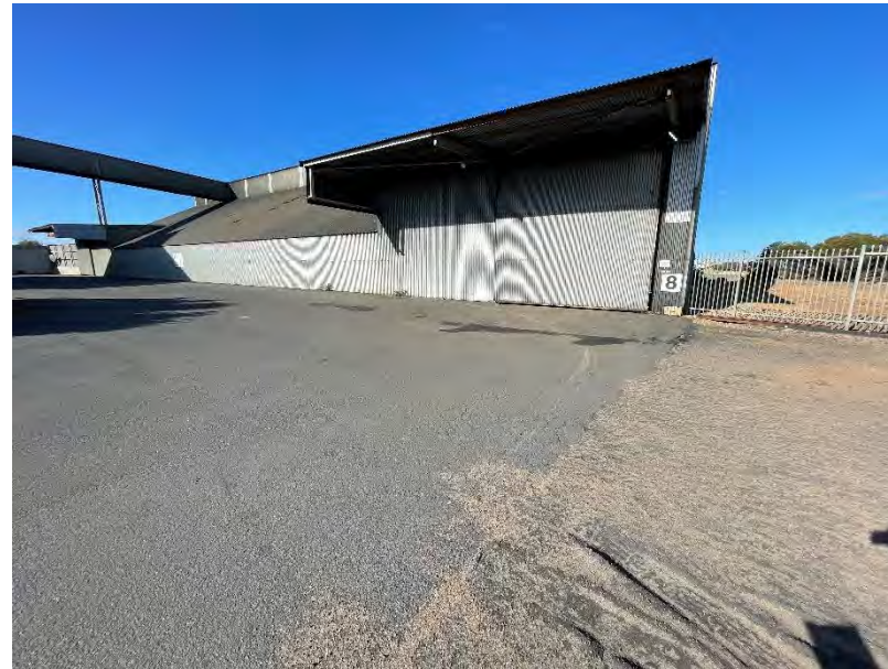
Photo 21: Damage on road edge and standing water in front of shed 8
