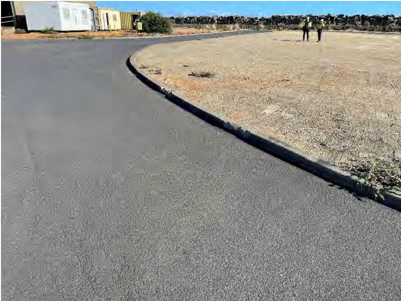
Photo 60: Damage to kerb
