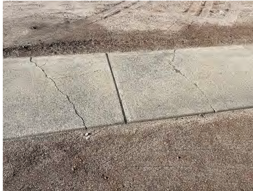
Photo 08: Cracks through the concrete path
