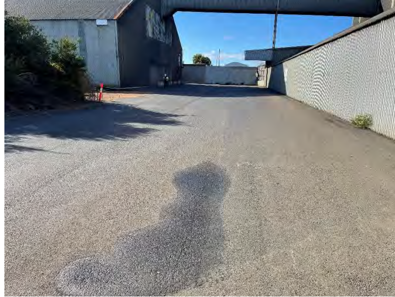
Photo 25: Wet road surface from roof shedding
