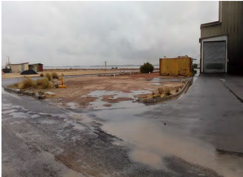
Photo 106: Localised ponding on the road
