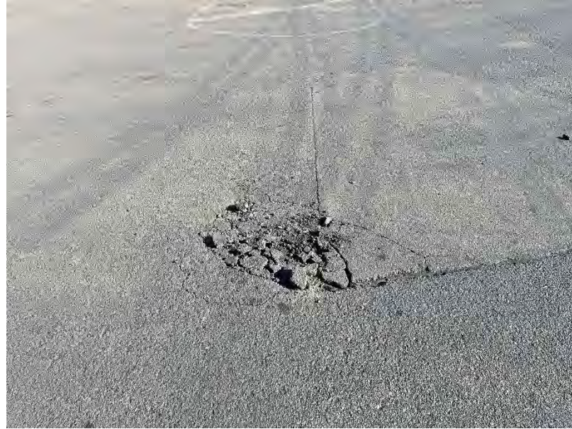
Photo 55: Damage to the road surface
