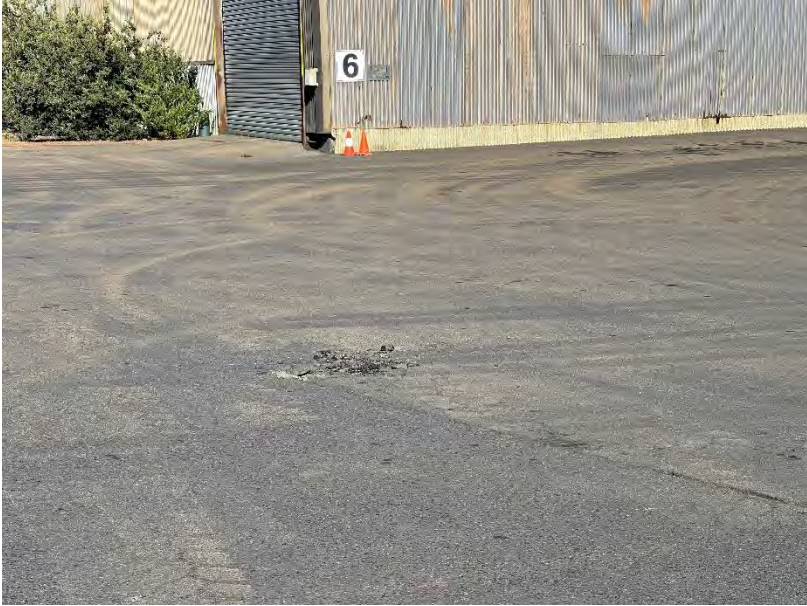
Photo 54: Damage to the road surface
