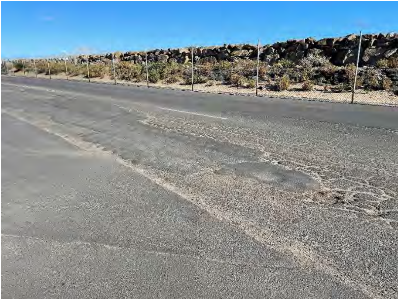
Photo 03: Outside of scope of works – full of cracks and pot-holes through the road
