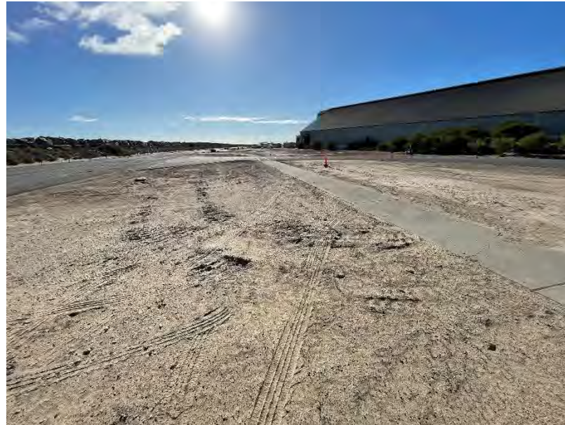
Photo 16: Cracks through the concrete path
