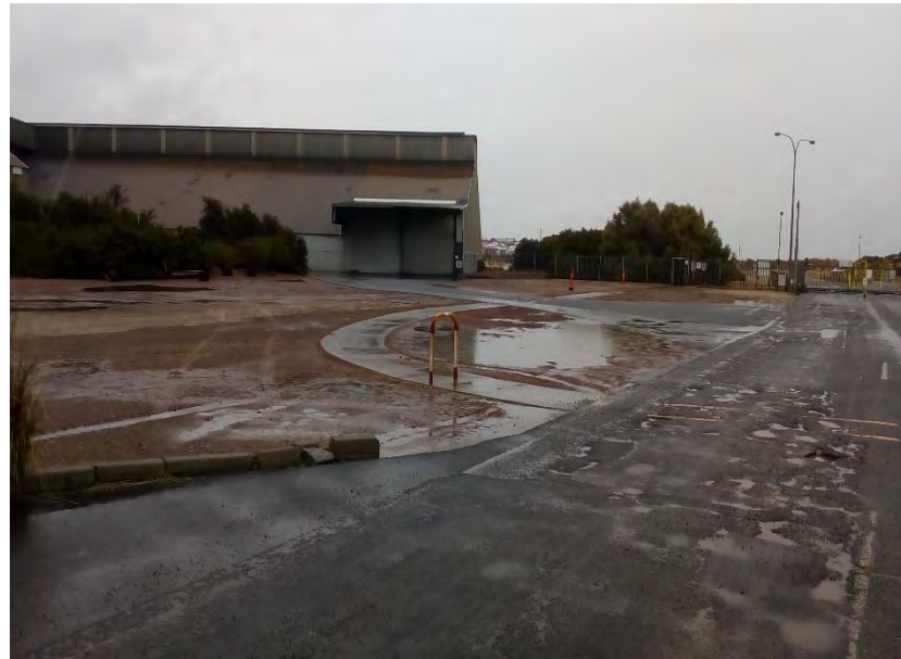
Photo 107: Localised ponding on verge
