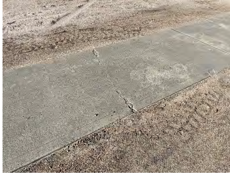
Photo 10: Cracks through the concrete path
