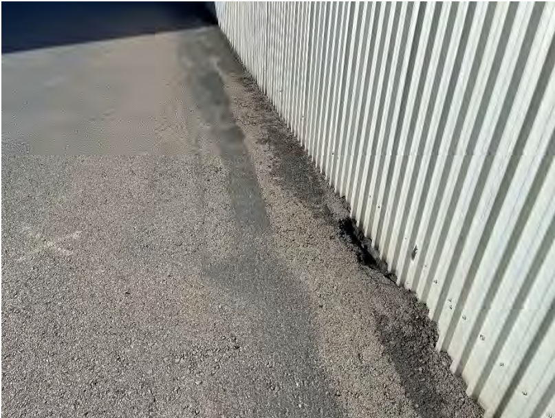
Photo 26: Damage to road edge
