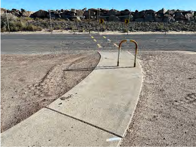
Photo 98: Grab rail requires refurbishment or consider removal.
