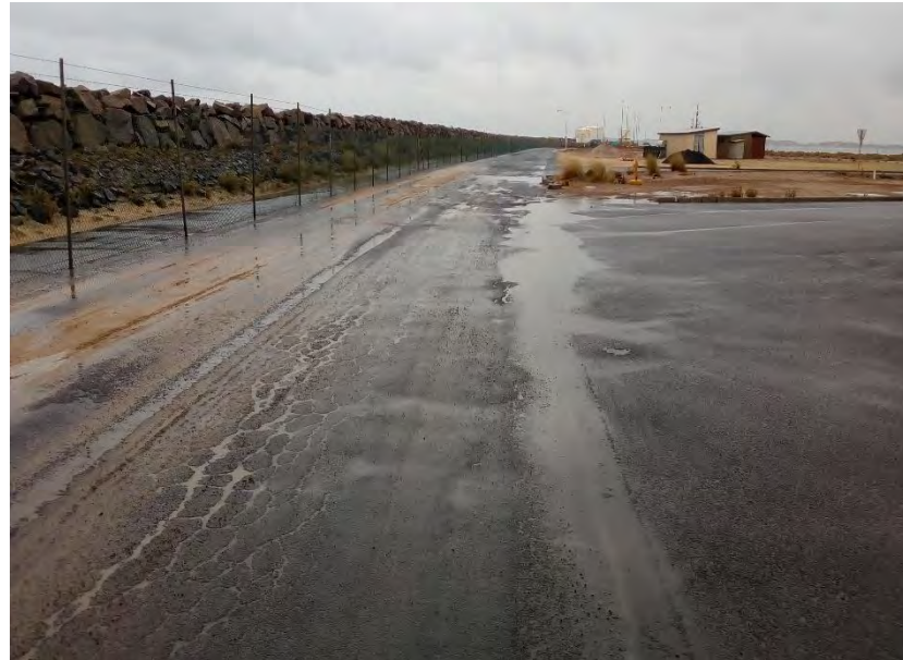
Photo 109: Localised ponding on the road
