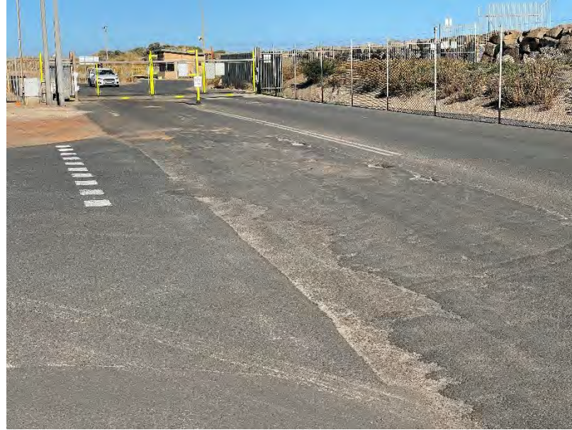
Photo 02: Outside of scope of works – full of cracks and pot-holes through the road
