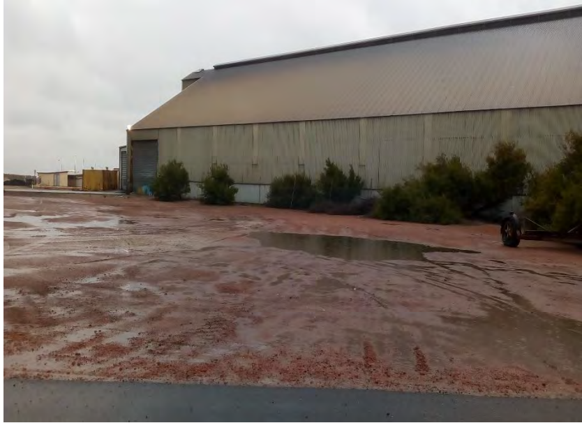
Photo 110: Localised ponding in verge
