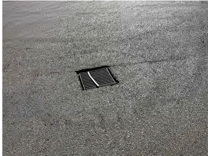
Photo 53: Damaged drainage pit
