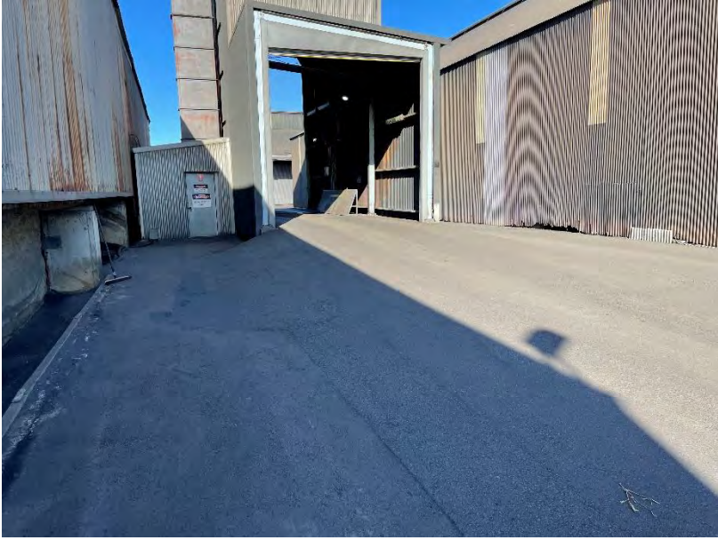
Photo 44: Steep slope at Shed 6
