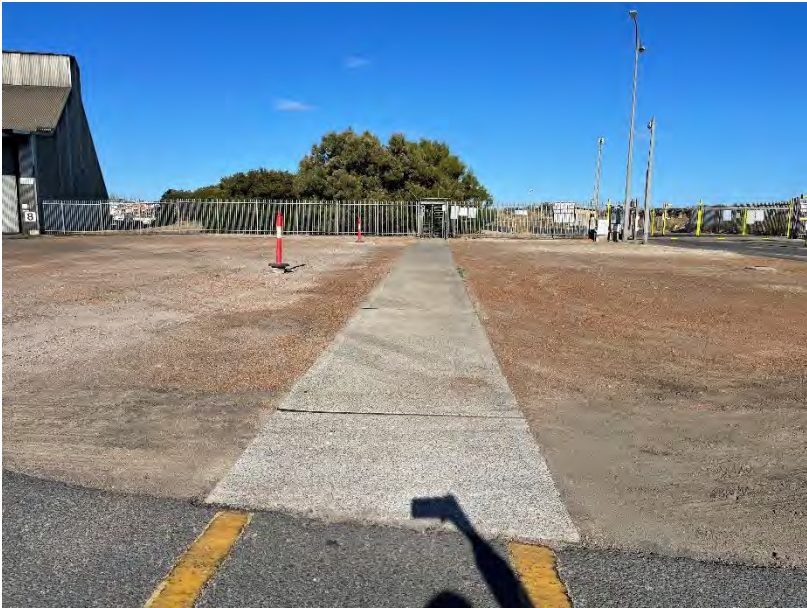
Photo 07: Cracks through the concrete path
