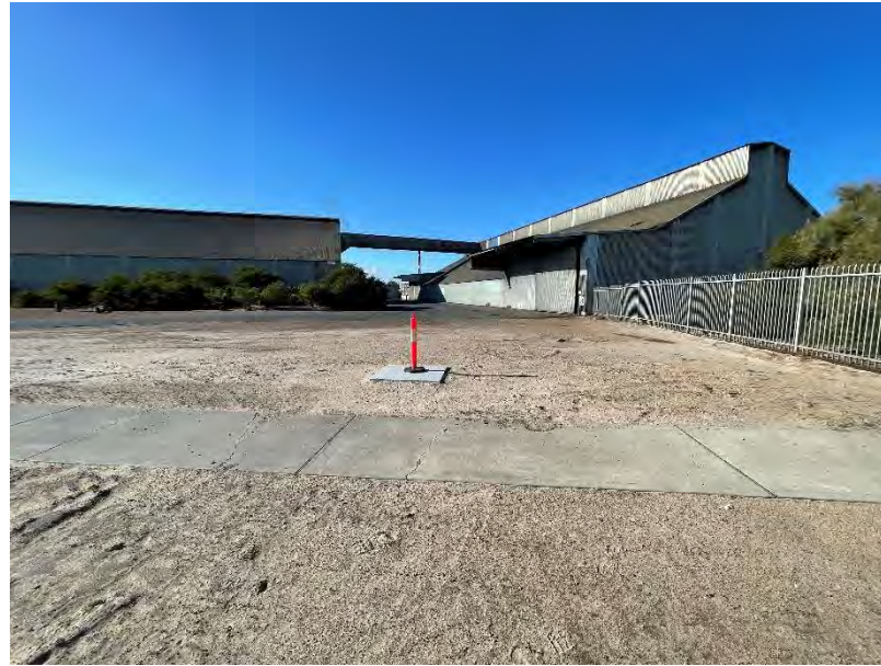
Photo 14: Cracks through the concrete path
