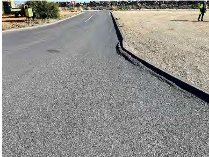
Photo 61: kerb and Road surface have moved
