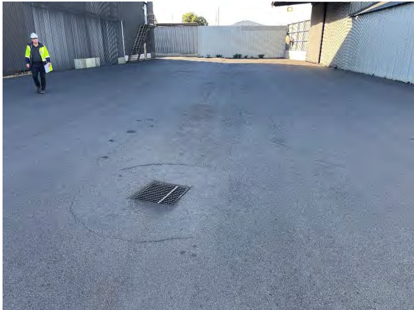
Photo 28: Settling around drainage pit
