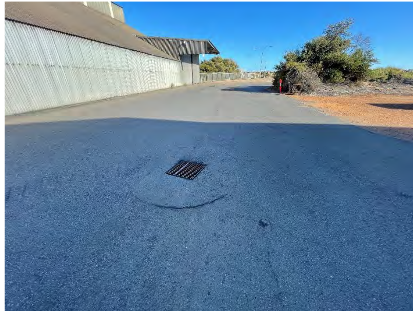
Photo 29: Settling around drainage pit
