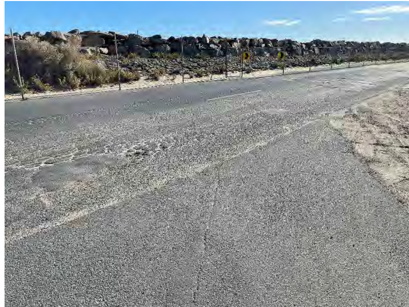
Photo 04: Outside of scope of works – full of cracks and pot-holes through the road
