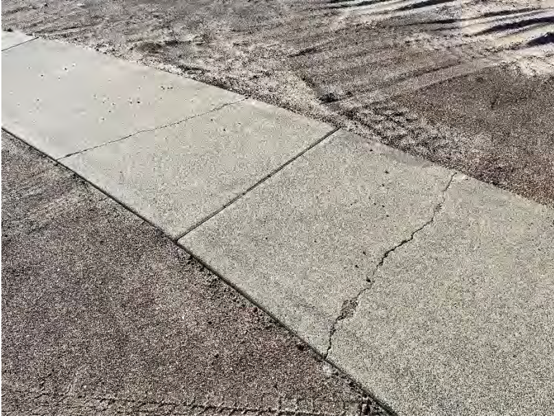
Photo 05: Cracks through the concrete path
