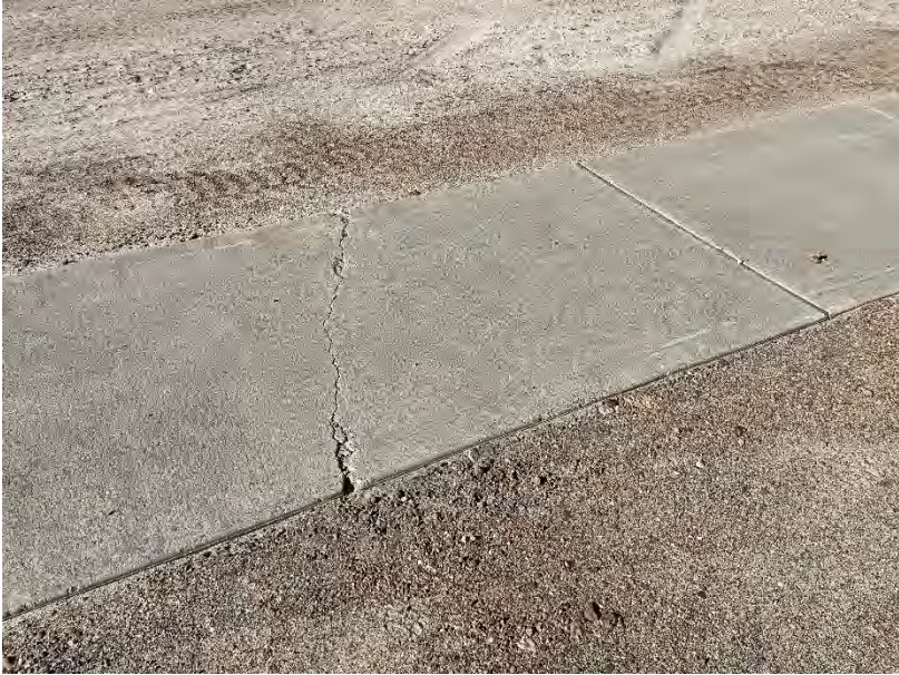
Photo 09: Cracks through the concrete path
