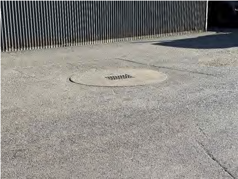
Photo 46: Surface grated inlet pit lid in good condition
