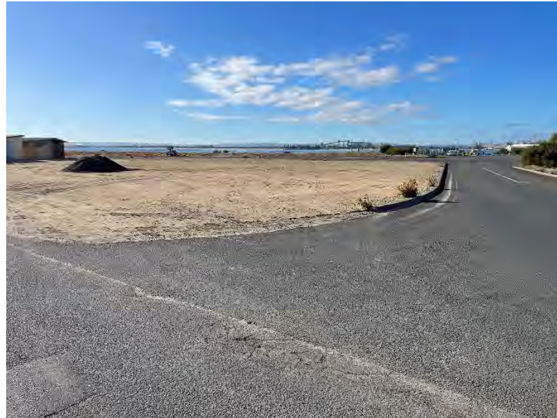
Photo 82: Missing kerb due to heavy vehicle sweeping through kerb
