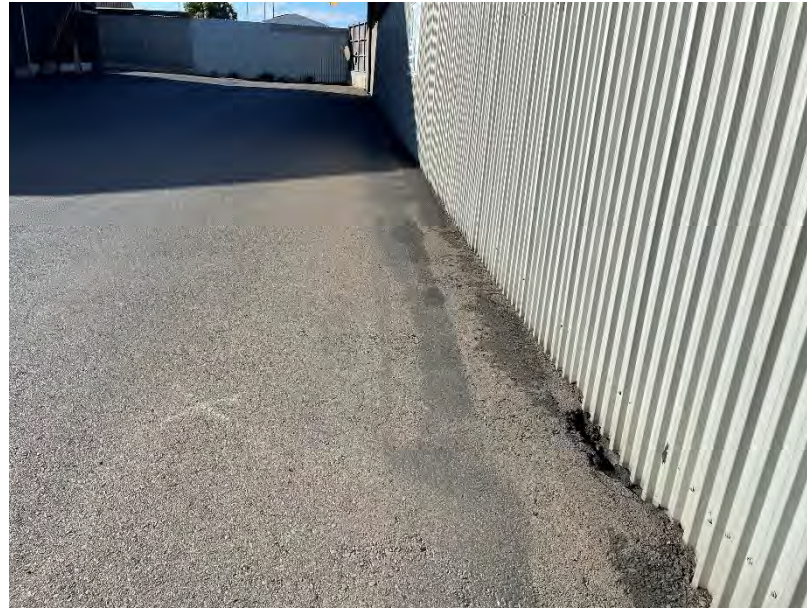
Photo 27: Damage to road edge
