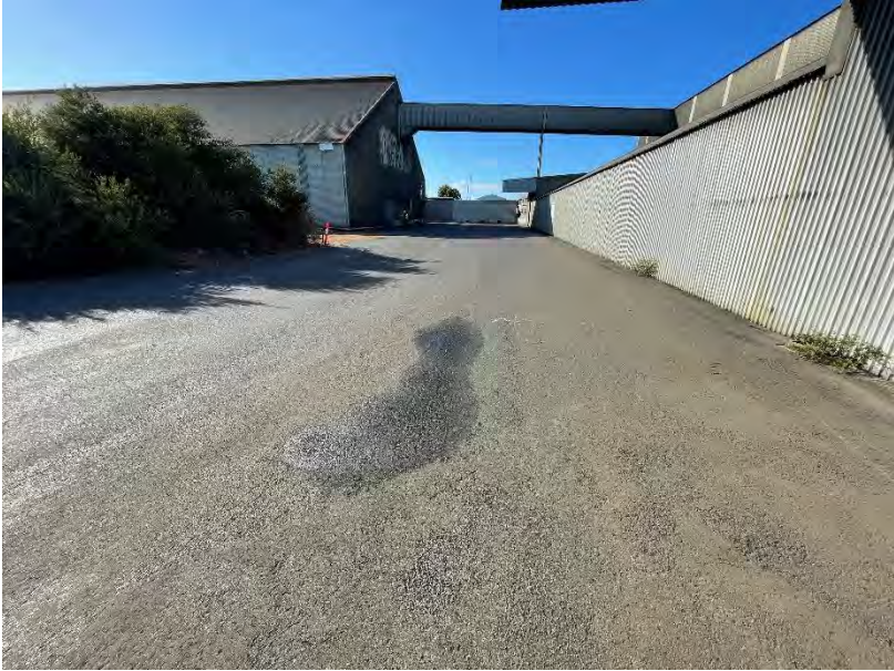
Photo 24: Wet road surface from roof shedding
