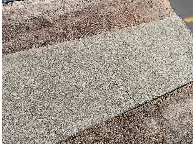
Photo 06: Cracks through the concrete path
