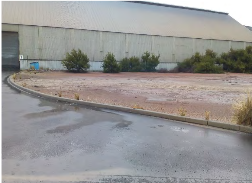
Photo 108: Localised ponding on road and verge
