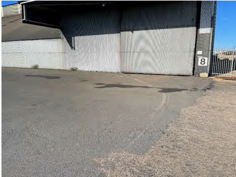
Photo 22: Damage on road edge and standing water in front of shed 8
