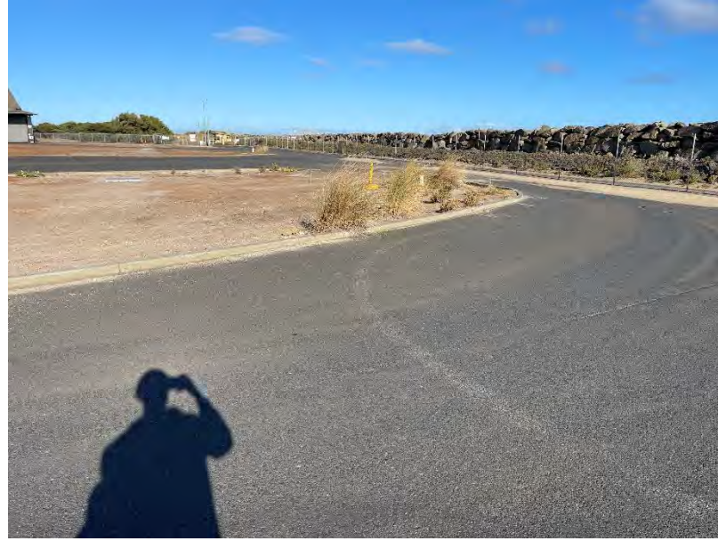
Photo 79: Damaged kerb due to heavy vehicle sweeping through kerb
