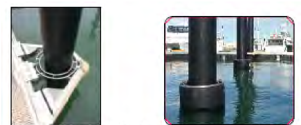
Figure 3: Typical Mooring Ring on Pile Guide (left) and Floating Mooring Ring (right)
