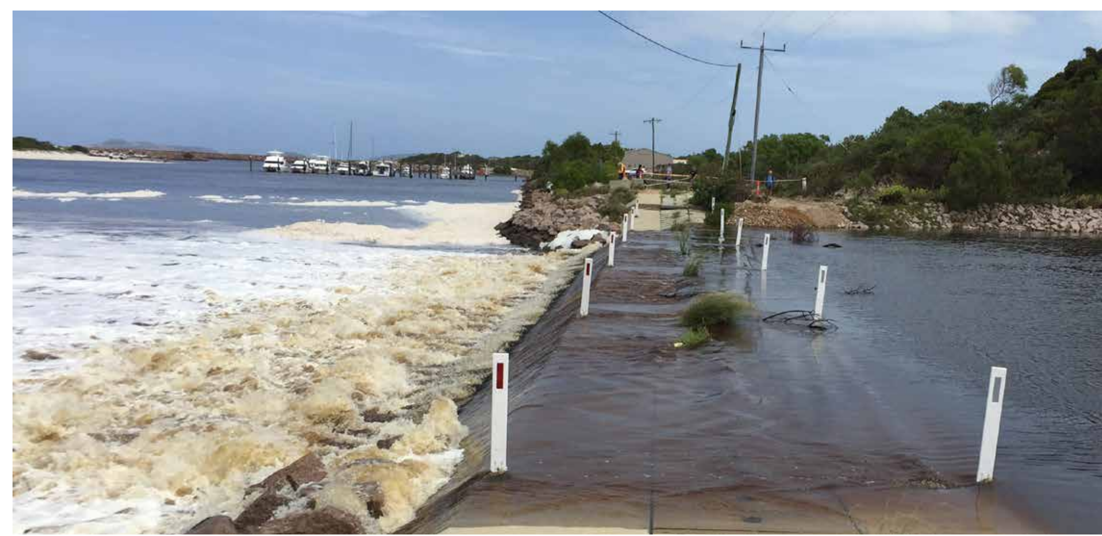
Bandy Creek Weir overtopping
